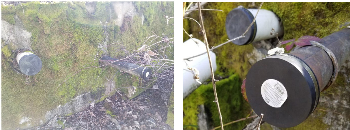
Figure 7. Basin D Stormwater SCMs (left: capped outfall STSOUT262 and STSOUT001057; right: capped outfall STSOUT263)
