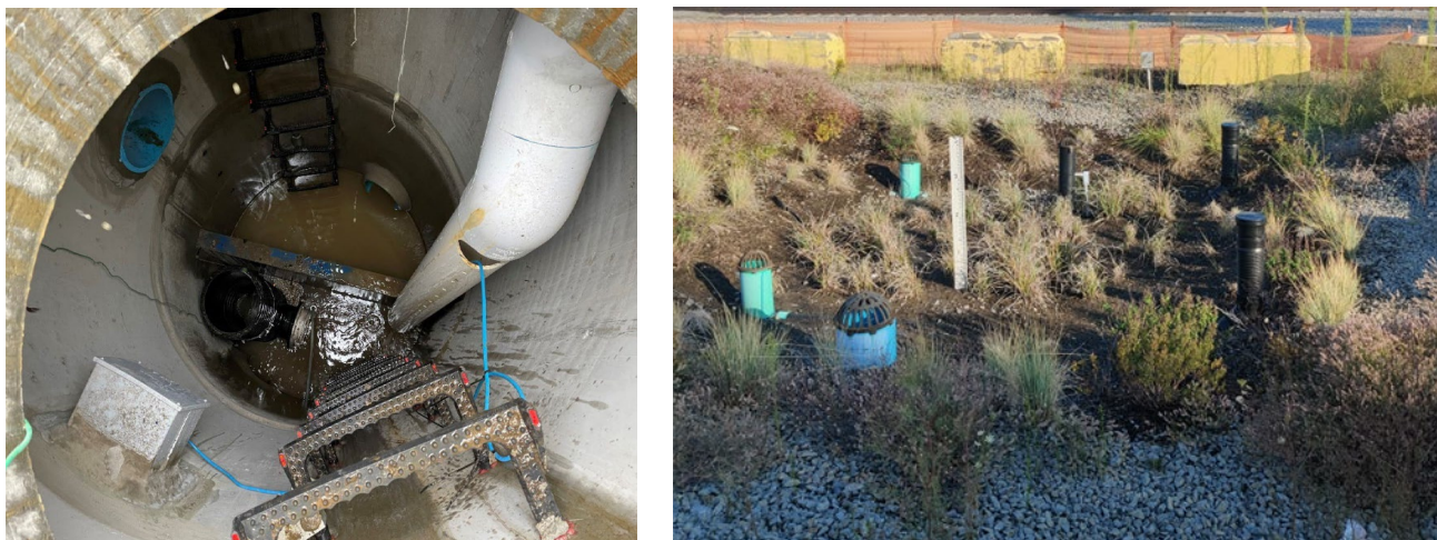
Figure 9. Basin K1 Stormwater SCMs (left: diversion manhole with pump; right: bioinfiltration basin)
