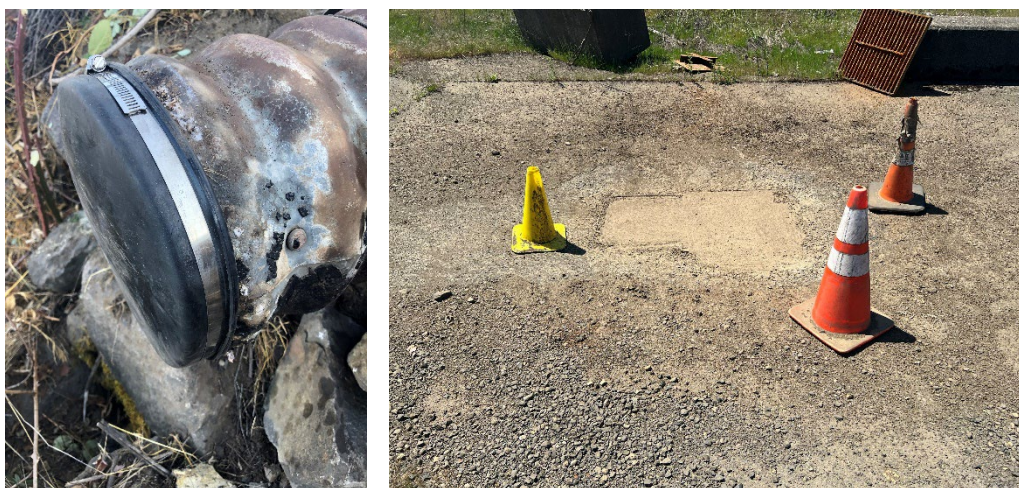
Figure 8. Basin J Stormwater SCMs (left: capped outfall; right: abandoned catch basin)
