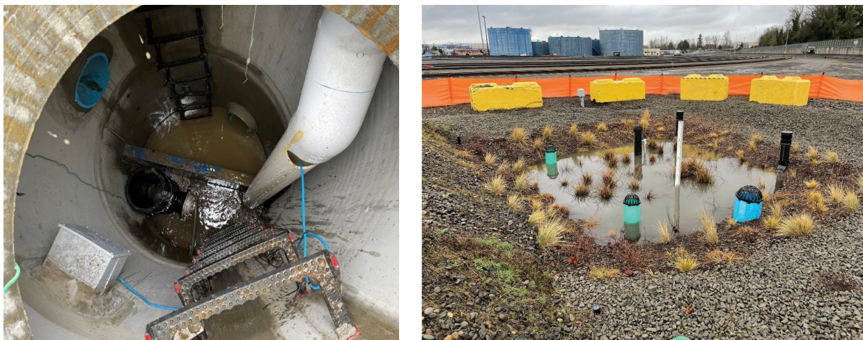
Figure 9. Basin K1 Stormwater SCMs (left: diversion manhole with pump; right: bioinfiltration basin)
