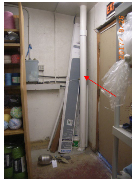
Interior view of SSV riser at southwest corner of suite 1220.
