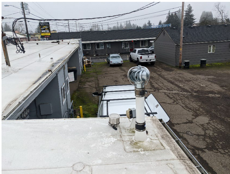
Wind-driven turbine on top of SSV riser above roof level – view facing south.
