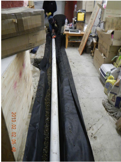
West SSV leg during installation – perforated 4-inch PVC bedded on gravel in a fabric-lined trench – view south.
