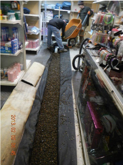
East SSV leg during installation – covered with gravel in a fabric-lined trench – view south.
