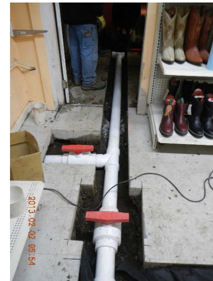
Collector line during installation. 1 st valve (foreground) controls the east leg, 2 nd valve (left of center) unused – view west.
