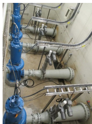
Wet Well/Dry Pit
