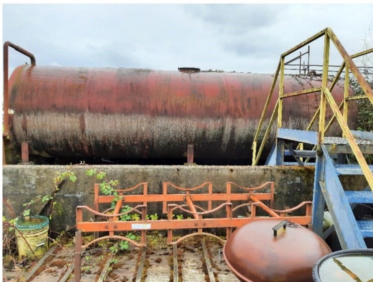
Photo 1: Outside, Above Ground Storage Tank (AST): Containers of used oil are pumped into this AST which is hard plumbed to the Industrial Boiler.
