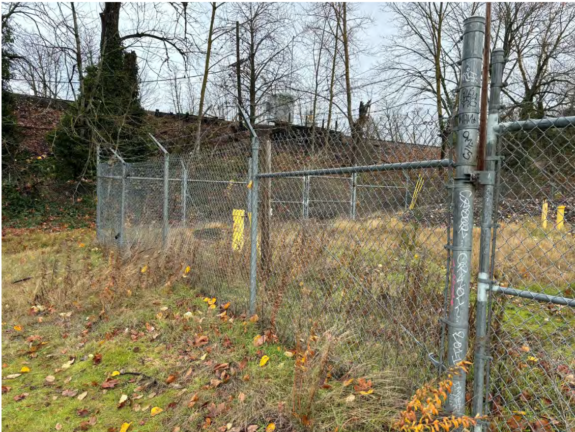
Photograph 8: Northwest corner fence requiring barbwire repair. View facing north.
