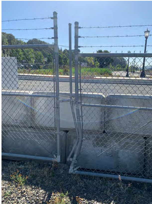
Photograph 6: Fence missing lock and chain. View facing south.
