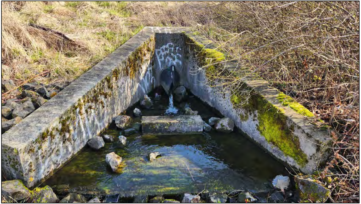
Photograph 5: Estimated 20 gpm flow from the stormwater outfall.
