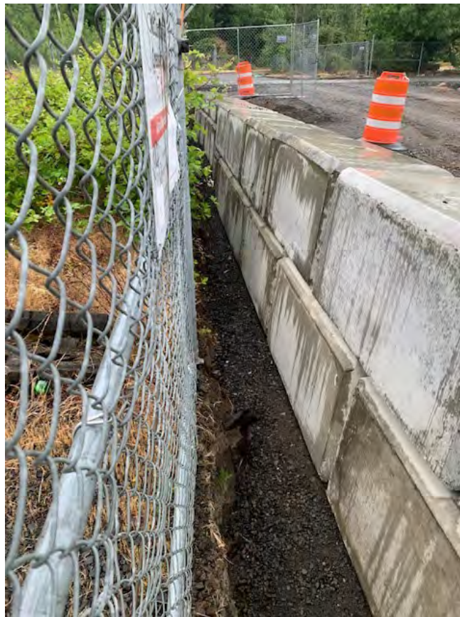
Photograph 8: Main site entry gate seen in Photo 7. Materials surrounding fence posts removed, potentially undermining fence posts. View facing east.
