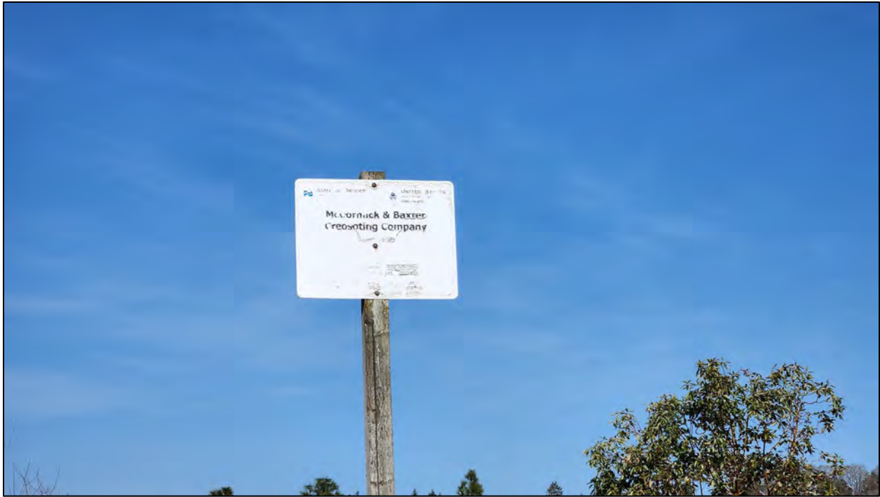
Photograph 7: Perimeter warning sign along fence on N. Van Houten that is faded and illegible and will require replacement.
