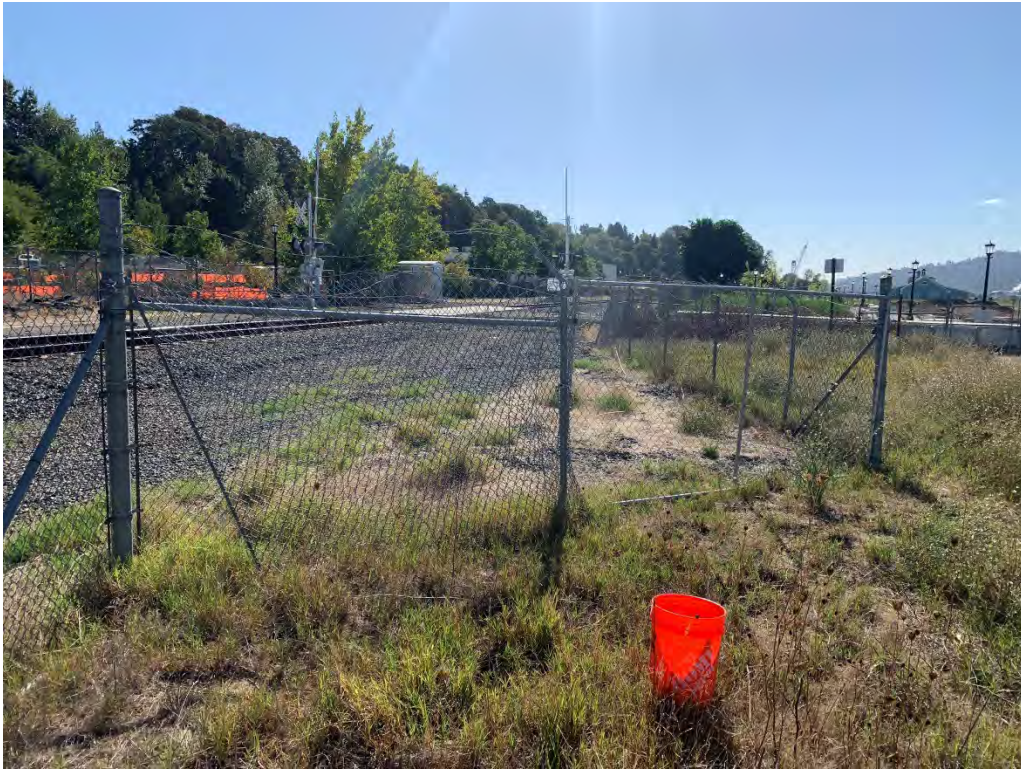
Photograph 7: Fence panel removed from southeast corner of Site. View facing south.
