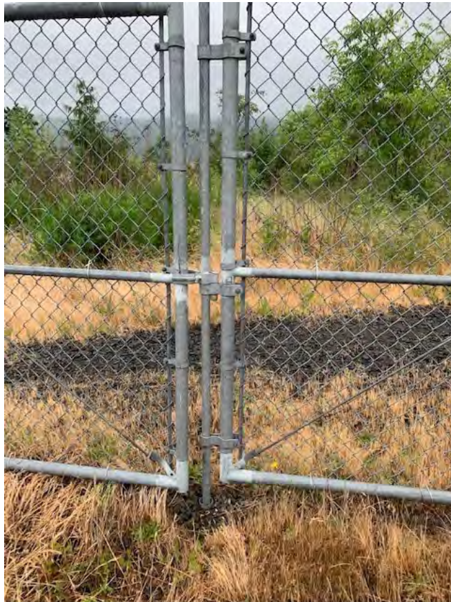
Photograph 6: Fence missing lock (replaced during site visit). View facing west.
