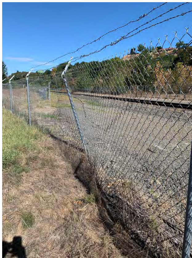
Photograph 8: Damaged fence post at southeast corner of Site. View facing east.
