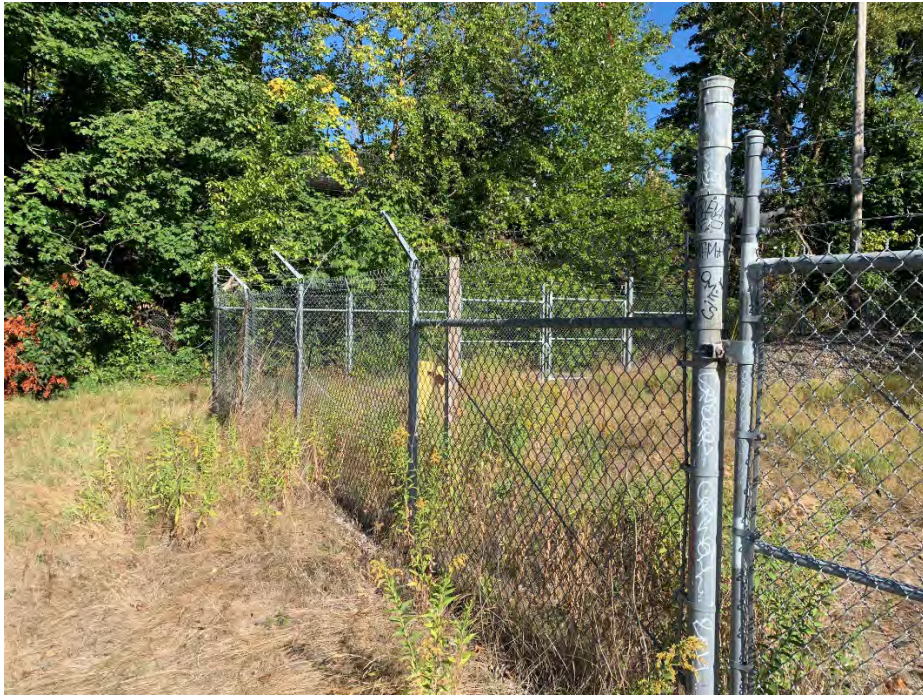
Photograph 9: Damaged barbed wire above fence at northwest corner of Site. View facing north.
