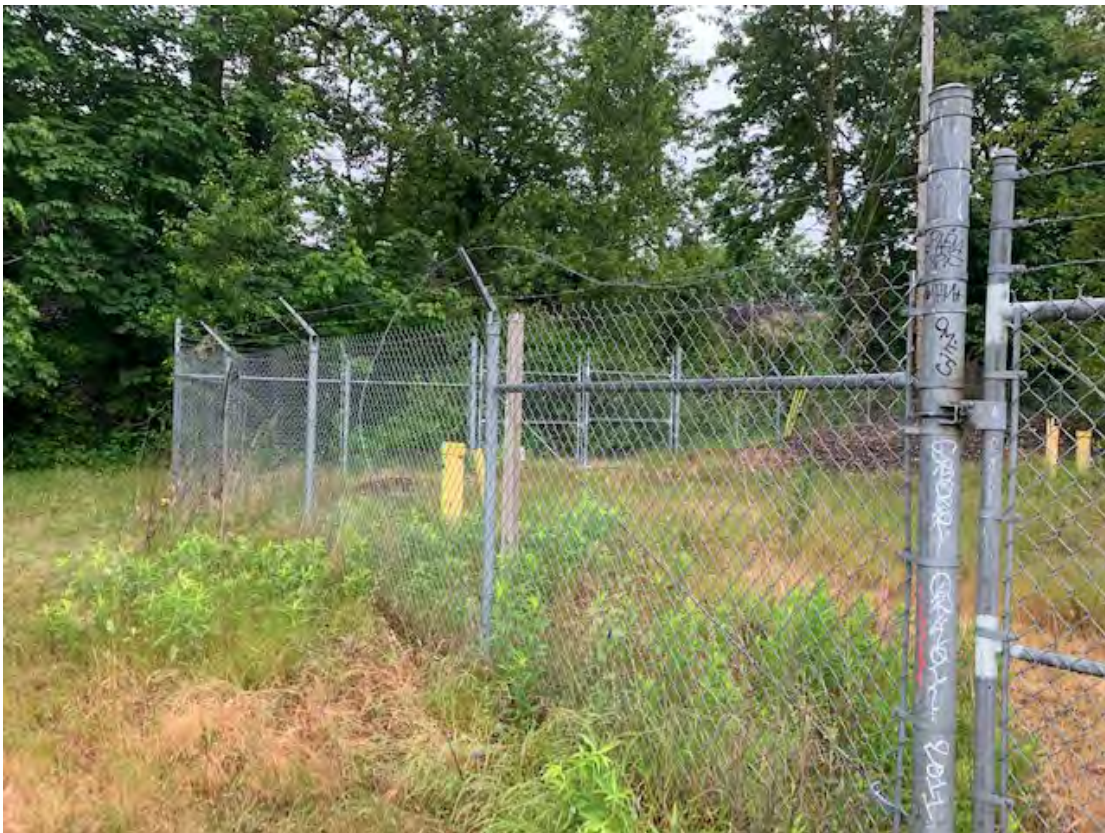
Photograph 4: Damaged barbed wire fence at northwest corner of site. View facing northeast.
