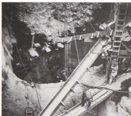
Two pot holes located at powerhouse site, to be filled with concrete.
