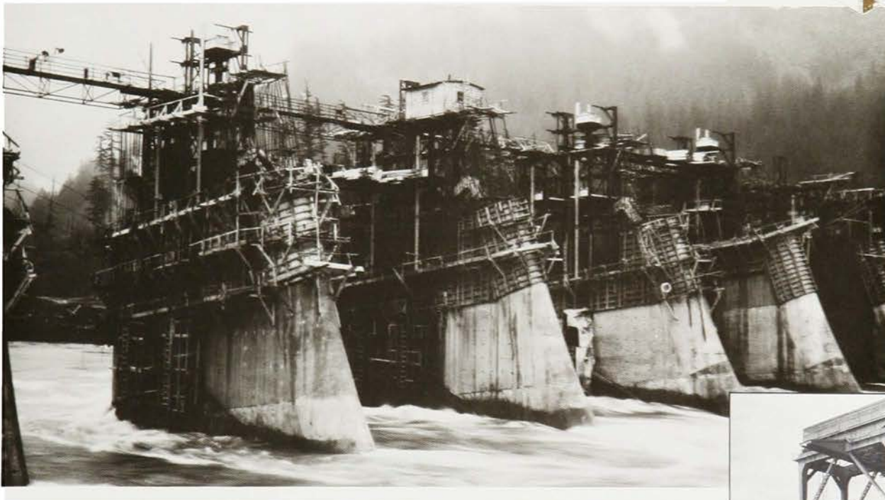
Downstream side of south half of spillway dam as workers finish piers.
