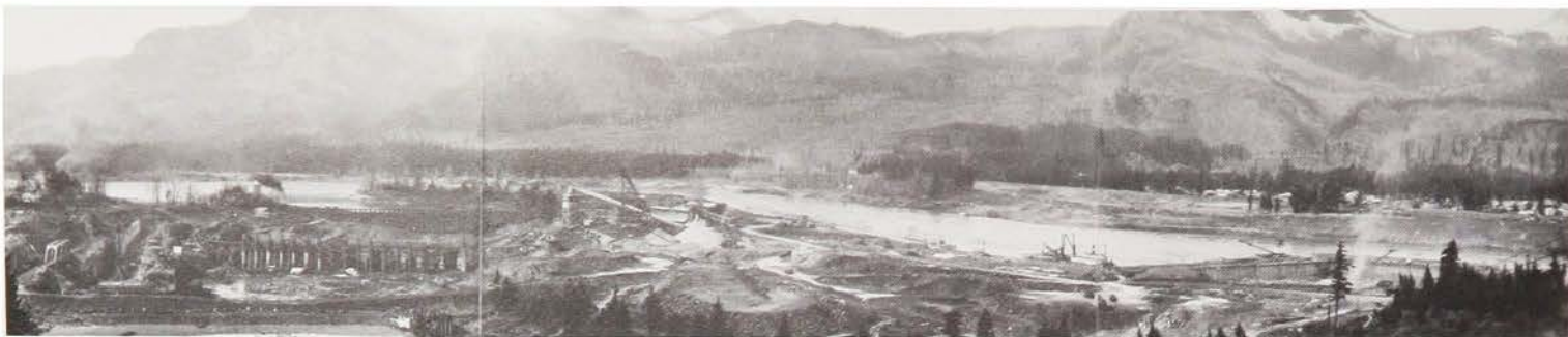
Panorama of Bonneville project with lock and original powerhouse nearly complete and spillway under construction.
