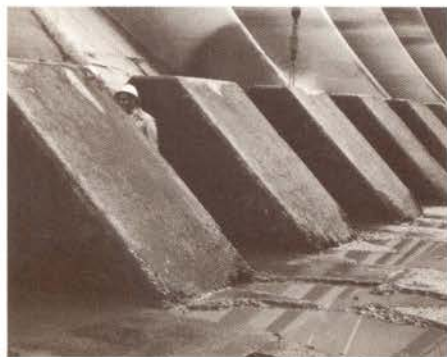
Detail of baffle deck showing concrete erosion after seventeen years.
