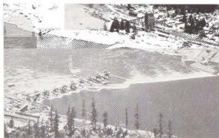
First step cofferdam has been removed allowing river to flow through piers. Bulkhead is in place. Third stage has been overtopped by flood waters.
