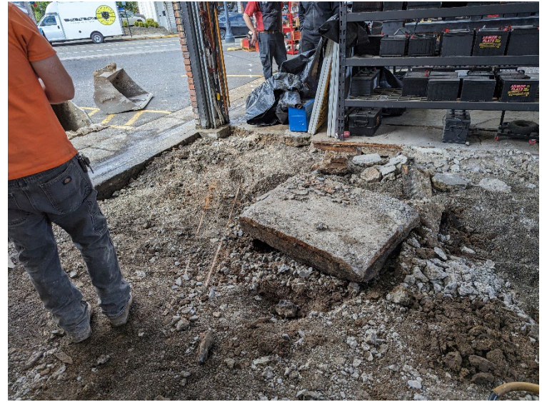
Exposed hydraulic lines under the concrete.
