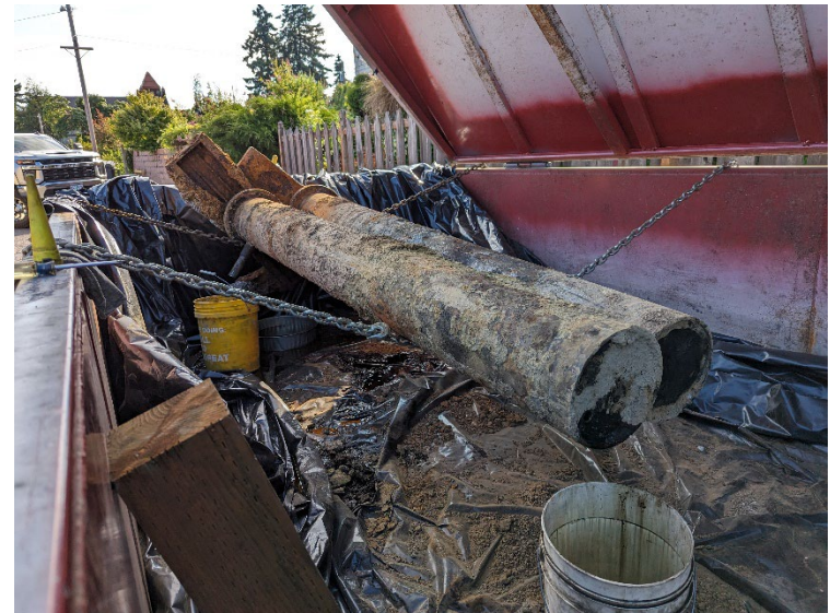
Hoist H01 and H02 stored over a plastic lined bin while draining residual oil.
