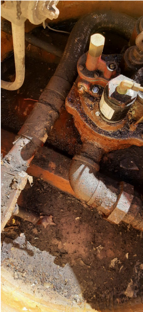
9: Regular sump turbine dripping product into sump
