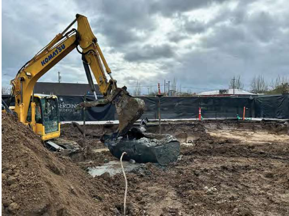
Photo 5. UST-03 was located to the south of UST-02. The tank was observed to contain gasoline-impacted water.
