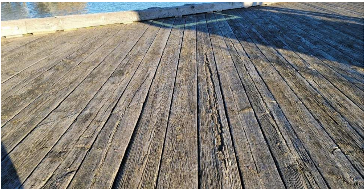
Picture 22. . Evidence of decay, riverside of service area.
