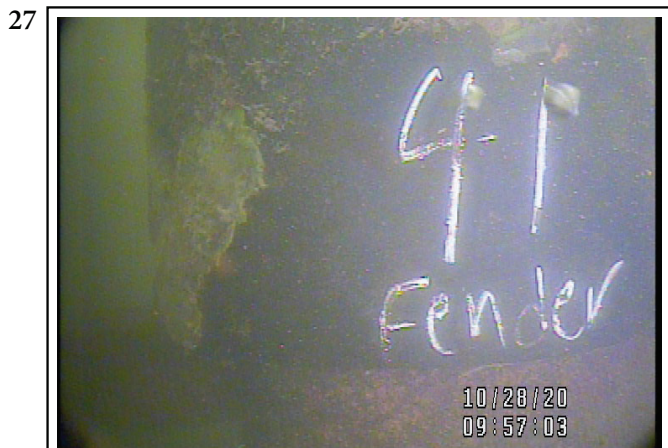
Fender Pile 41 - Minor corrosion sighted.
