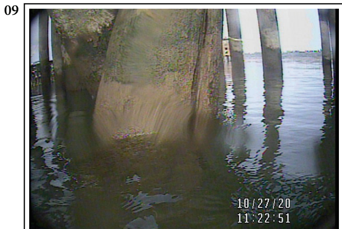
Pile 50 B - Splitting observed.
