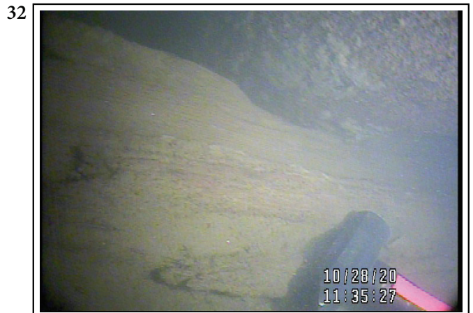
Pile 41 B - Loose at top. No splitting observed at mudline.
