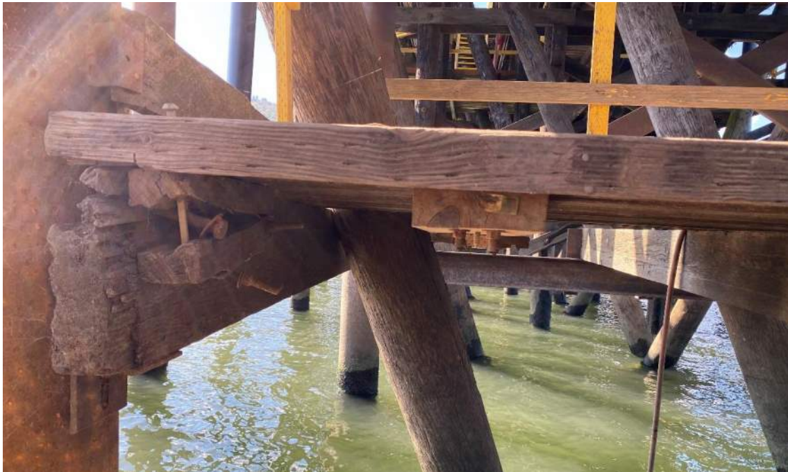
Picture 34. Grid 46, lower platform to floating deck, upstream side. Note significant framing decay and failing connection.
