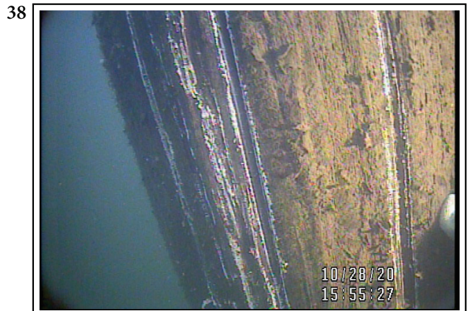
Pile 32 D - Splitting observed.
