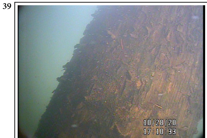
Pile 32 D - Weather checking observed.
