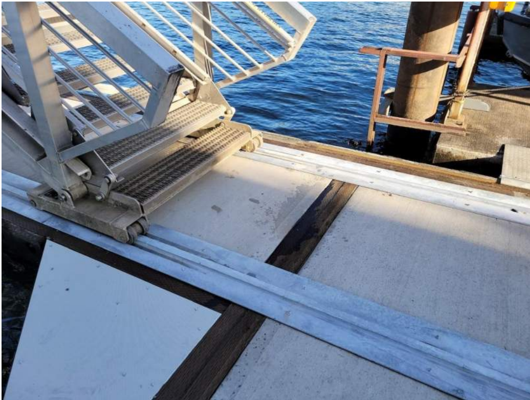
Picture 40. Gangway landing and guides (2021).
