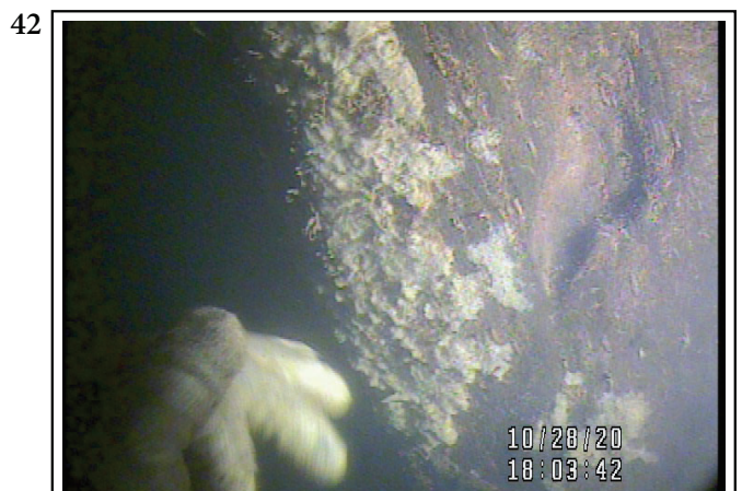
Pile 32 D - Pocket of wood missing observed.
