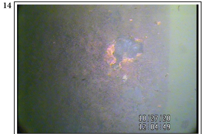
Fender Pile 48 - Minor corrosion sighted.
