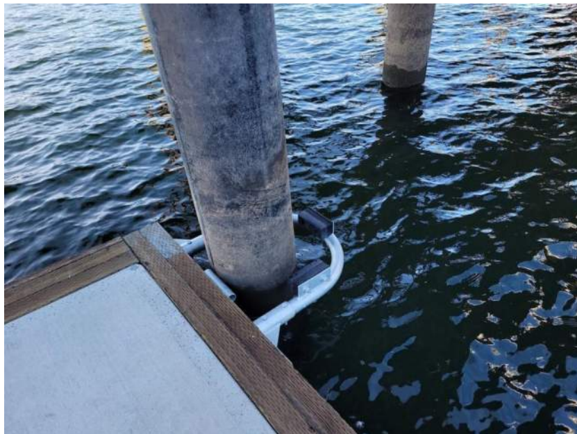
Picture 43. Gangway landing (2021). Typical guide system.
