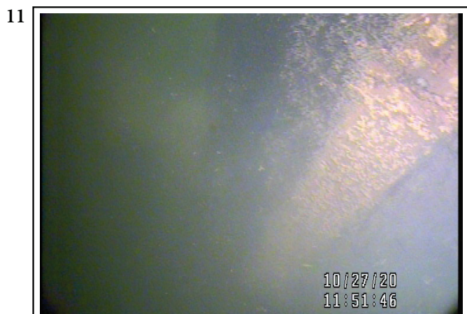
Pile 49 - Minor corrosion sighted.
