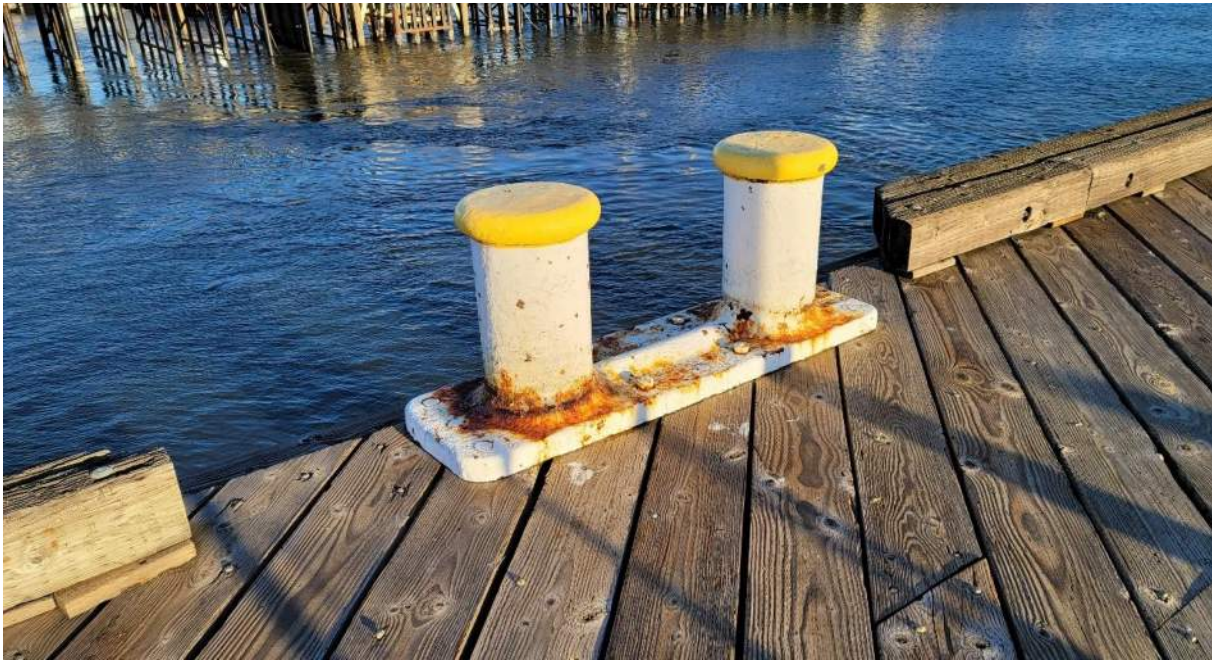
Picture 19. Bollard 'C'. Note wear to coating from line abrasion.
