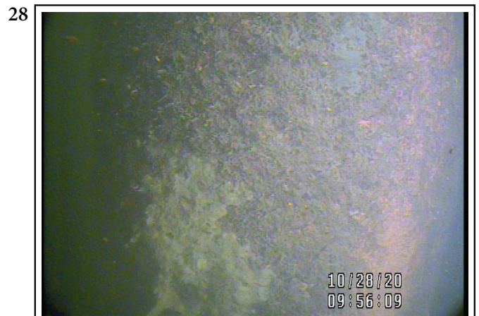
Fender Pile 41 - Minor corrosion sighted.
