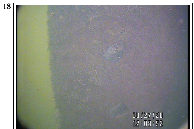
Pile 47 E - Minor corrosion sighted.
