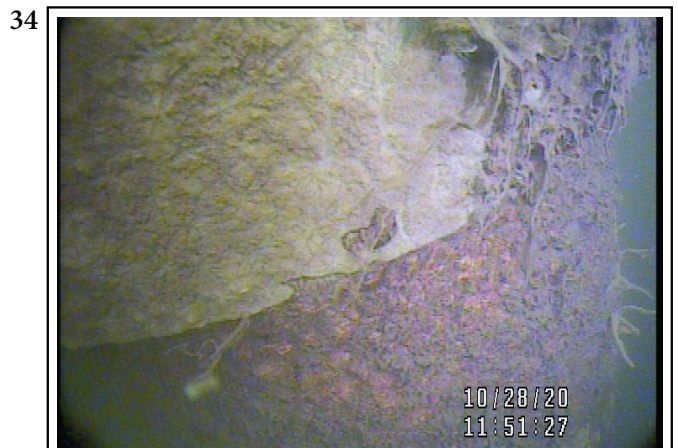
Fender Pile 38 - Minor corrosion sighted.
