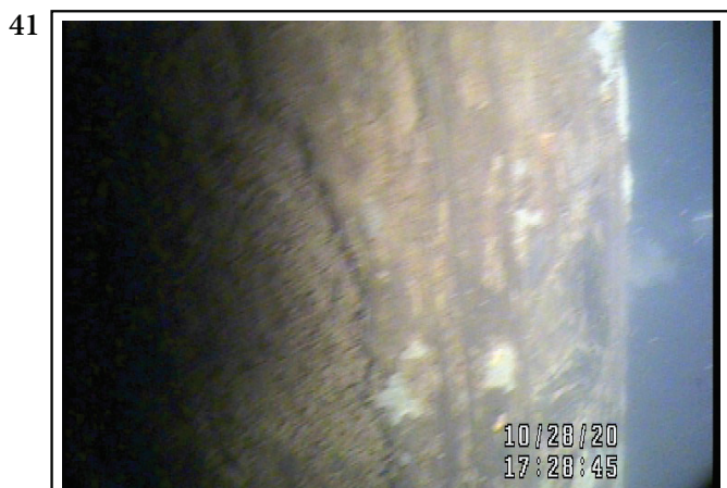
Pile 32 D - Pocket of wood missing observed.
