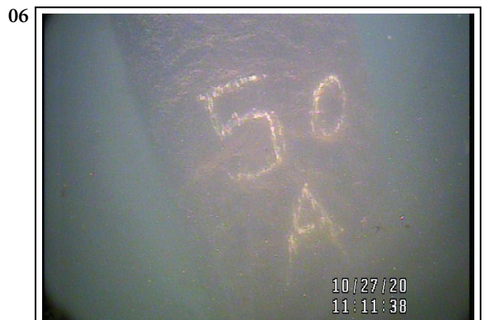
Pile 50 A - Loose at top.
