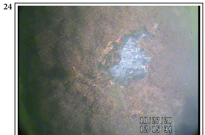
Pile 47 A - Minor corrosion sighted.
