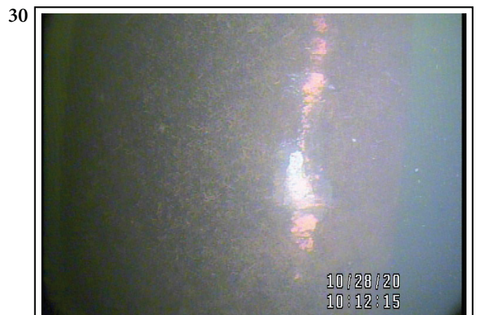
Fender Pile 41 Downstream side - Minor corrosion sighted.
