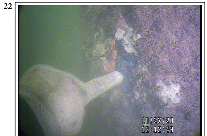
Pile 47 B - Minor corrosion sighted.
