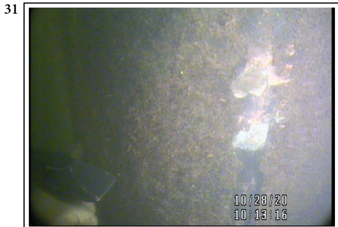
Pile 41 B - Loose at top.
