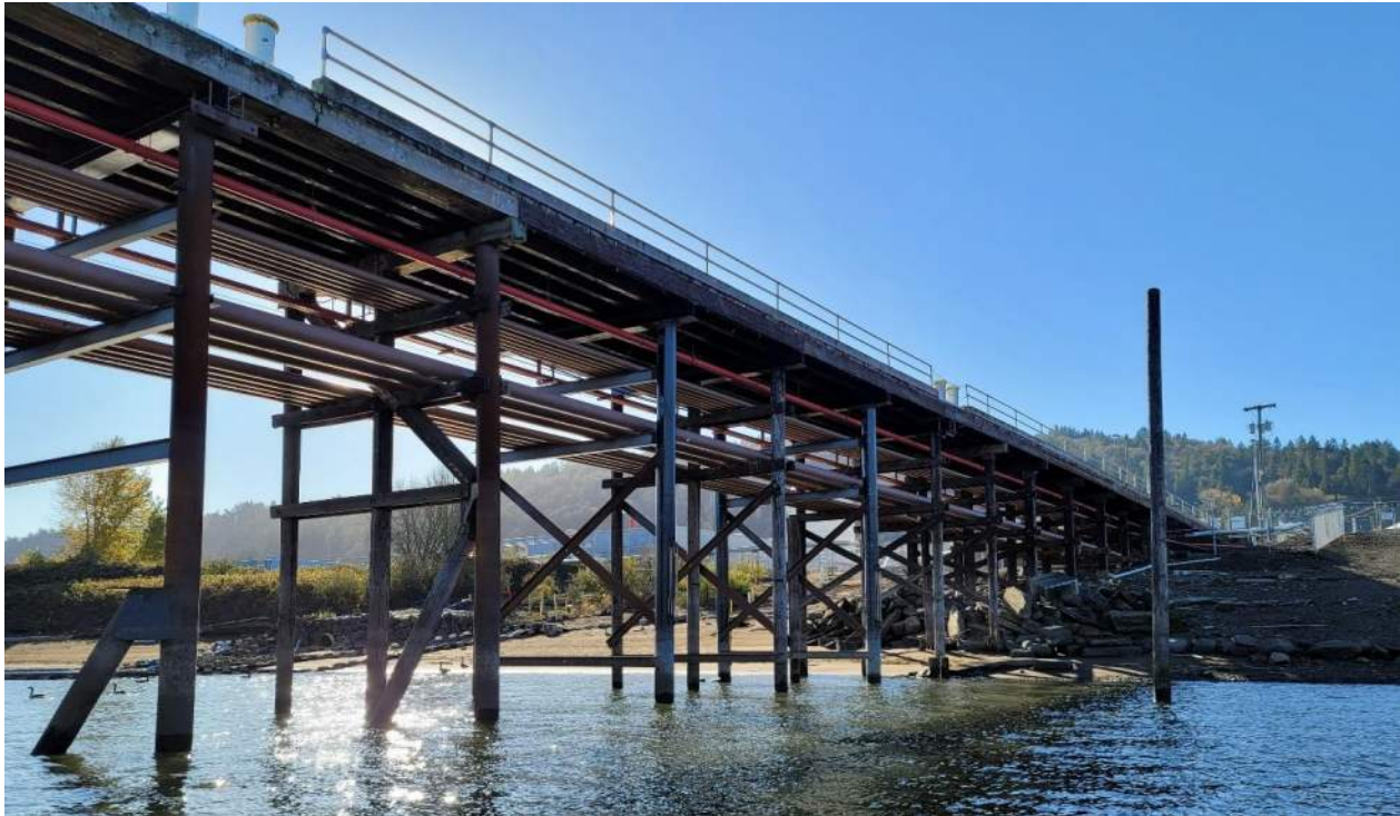
Picture 3. Pier approach from the downstream side. Note the combination of steel piles and bracing with the original timber elements.
