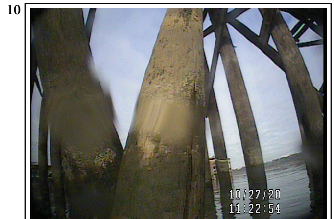
Pile 50 B - Splitting observed.
