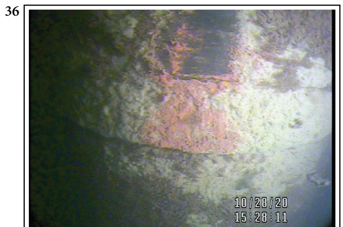
Fender Pile 33 - Minor corrosion sighted.
