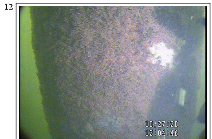
Pile 49 - Minor corrosion sighted.
