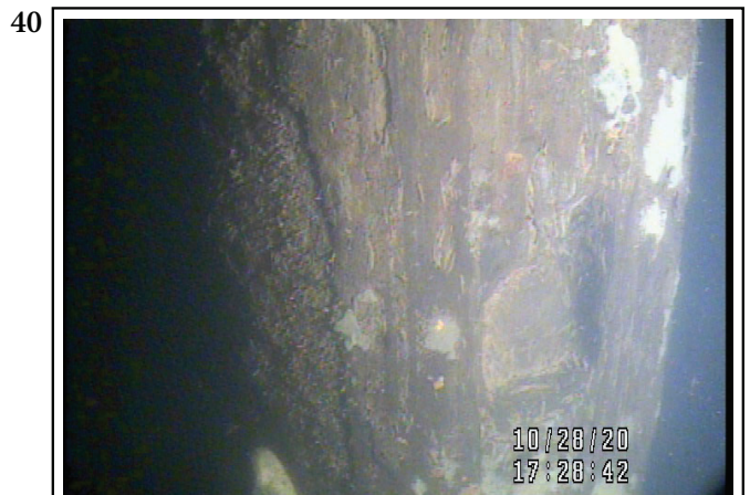
Pile 32 D - Pocket of wood missing observed.
