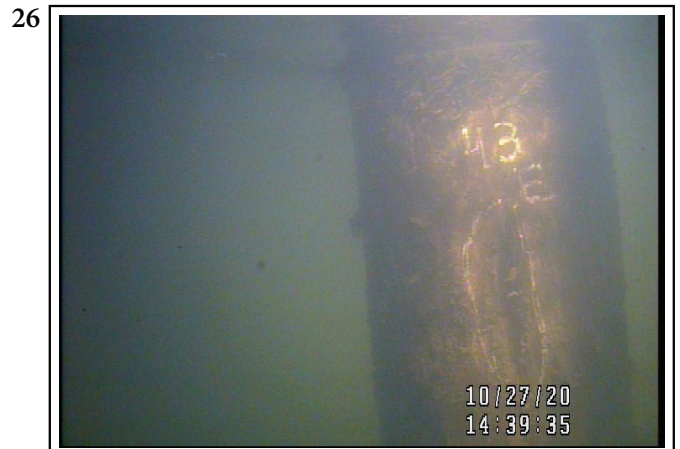
Pile 43 E - Timber compromise observed.
