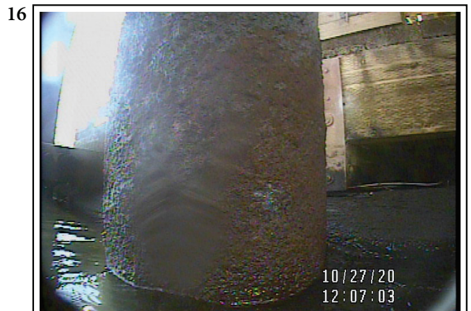
Fender Pile 47 - Minor corrosion sighted.
