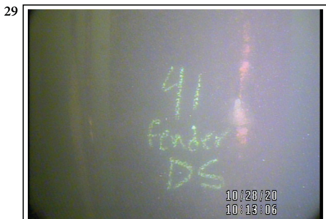
Fender Pile 41 Downstream side - Minor corrosion sighted.
