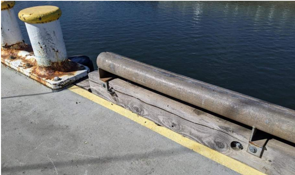
Picture 25. Split in bullrail, downstream berth.
