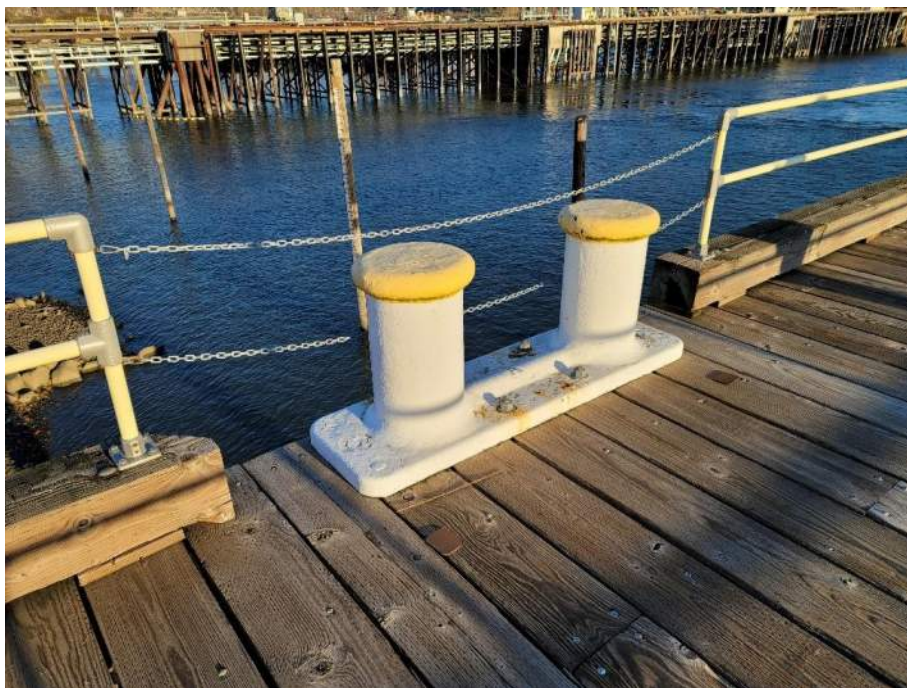
Picture 18. Bollard 'A', deck, handrails along approach. It does not appear to see regular use.
