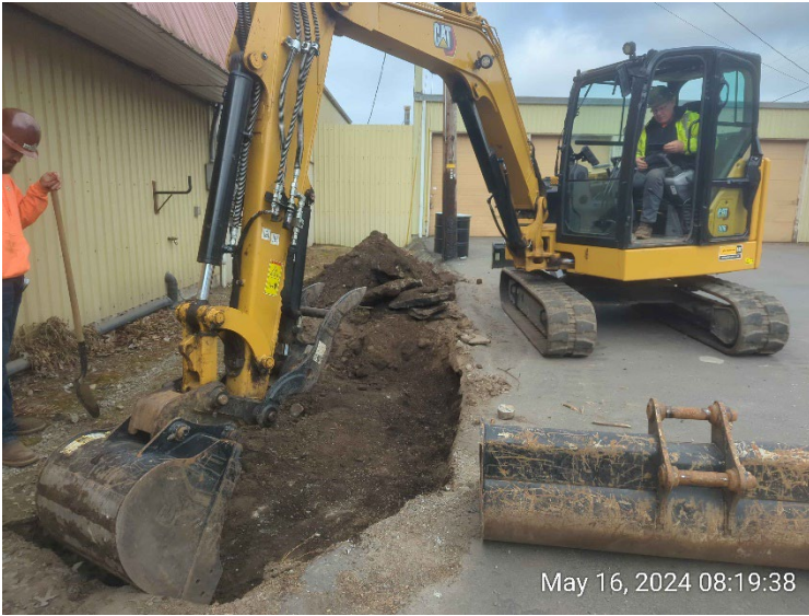
An excavator was used to expose the abandoned septic tank on the north side of the site building.
