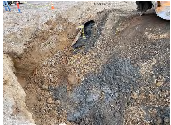
Photo #2 Stained soil in tank pit.
