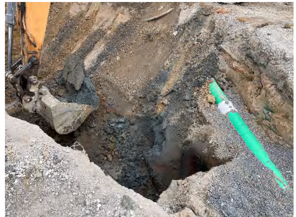
Photo #4 Stained soil and sewer line. Removing visually impacted soil.
