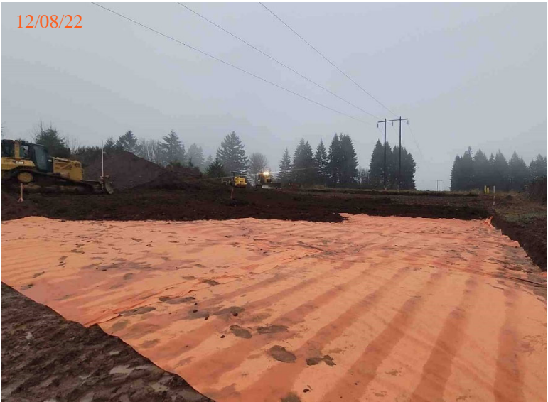
Placing a 3-foot-thick clean soil cap in 1-foot-lifts over demarcation fabric and compacting with a sheep's foot roller.
