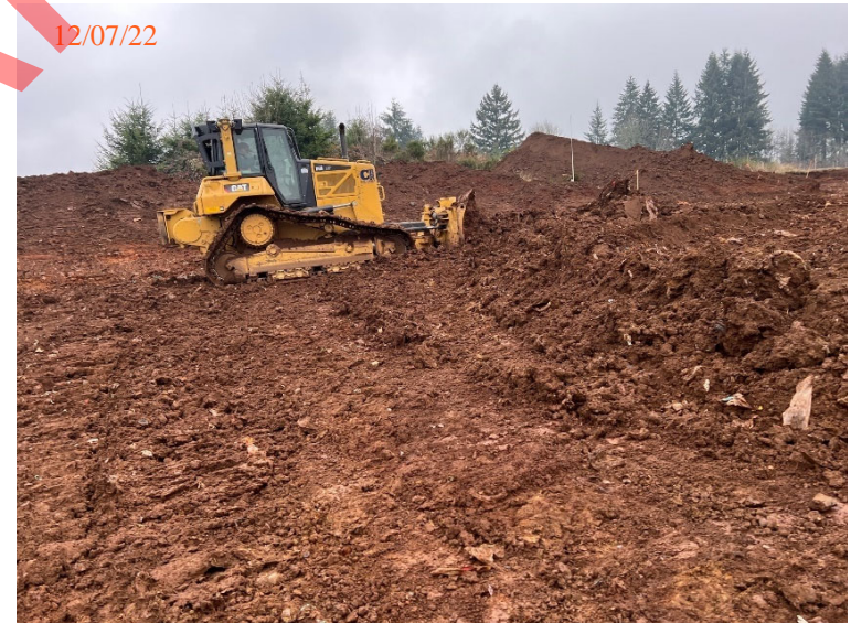
Reconsolidating solid waste in the northern portion of the USWDC – view west.
