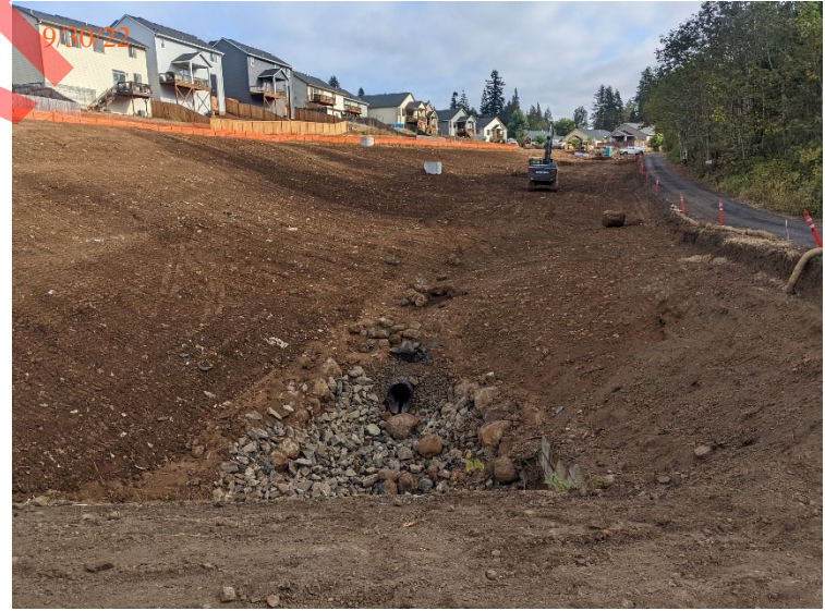
View east of completed storm-water dissipation pad, storm sewer outfall, subgrade channel, and manholes.
