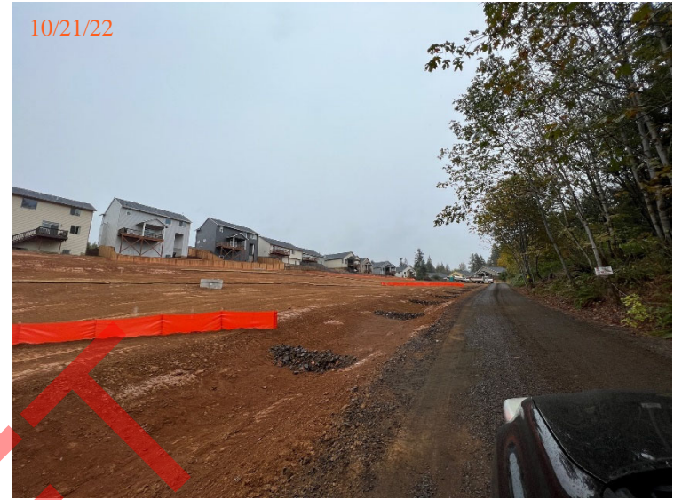
3-foot clean soil cap placed over the entire FSWDA – View northeast of channel next to Barrick Ln.
