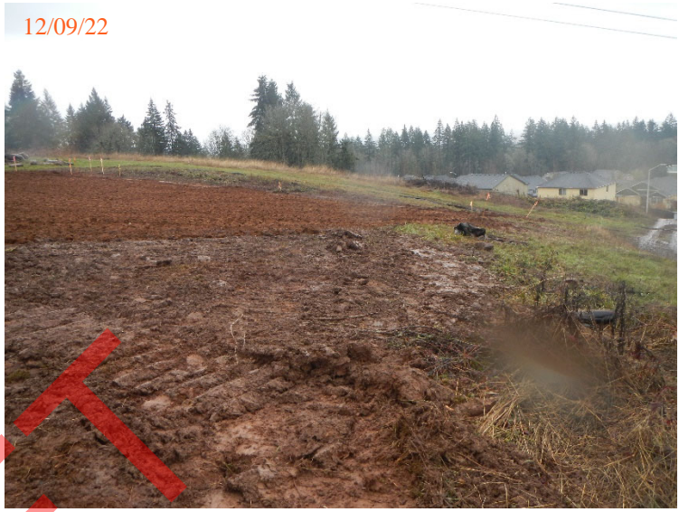
View of the southern portion of the USWDC following placement of a 3-foot-thick soil cap.
