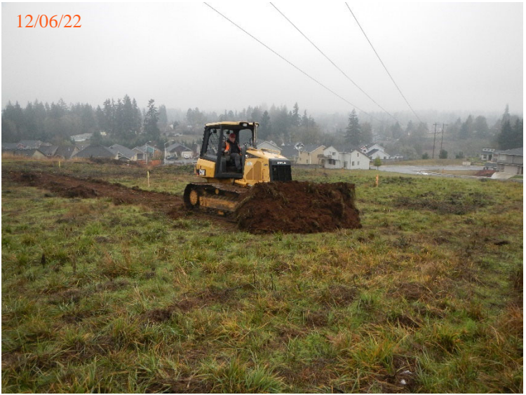
Removing the existing cap soil from USWDC – view southwest and stockpiling for later reuse.
