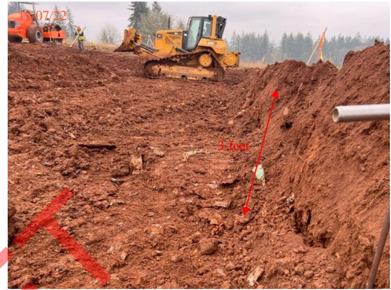
Reconsolidating solid waste prior to capping – southern portion of USWDC, view east.
