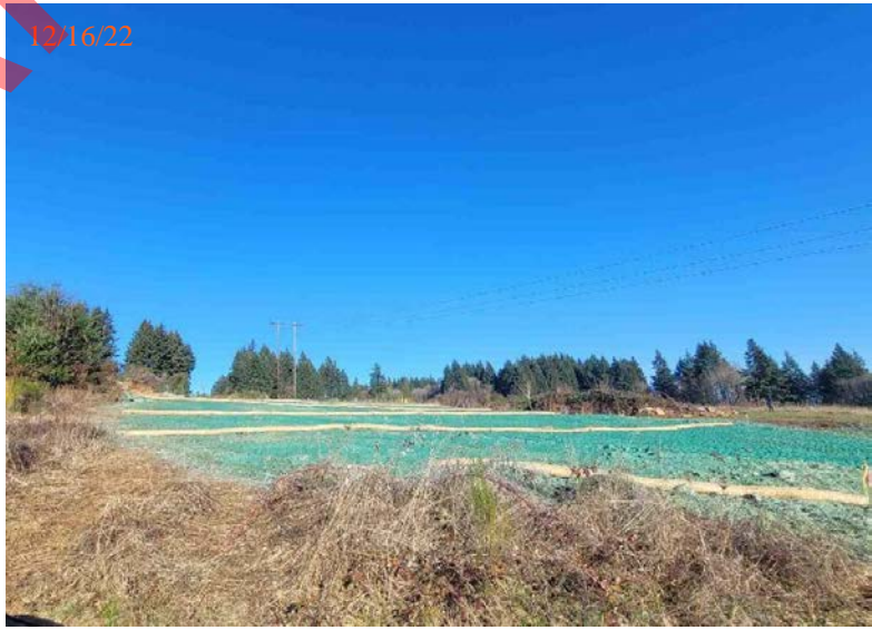
View of USWDC following application of hydro-mulch and installation of straw wattles perpendicular to slope.
