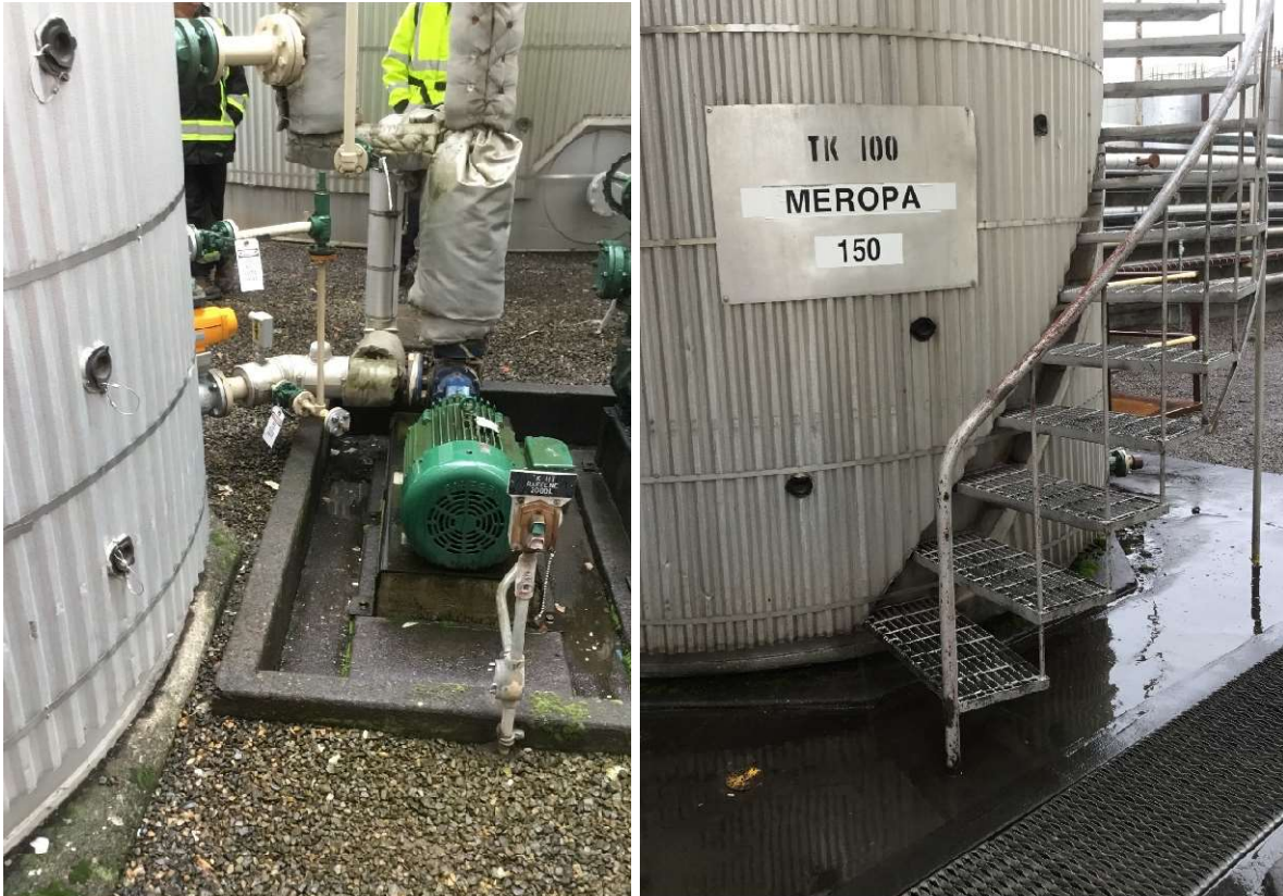
Figure 7-1: Example Over-Constrained Conditions Left: Short pipe run to anchored pump at Tank 117 Right: Anchored stair handrail at Tank 100
