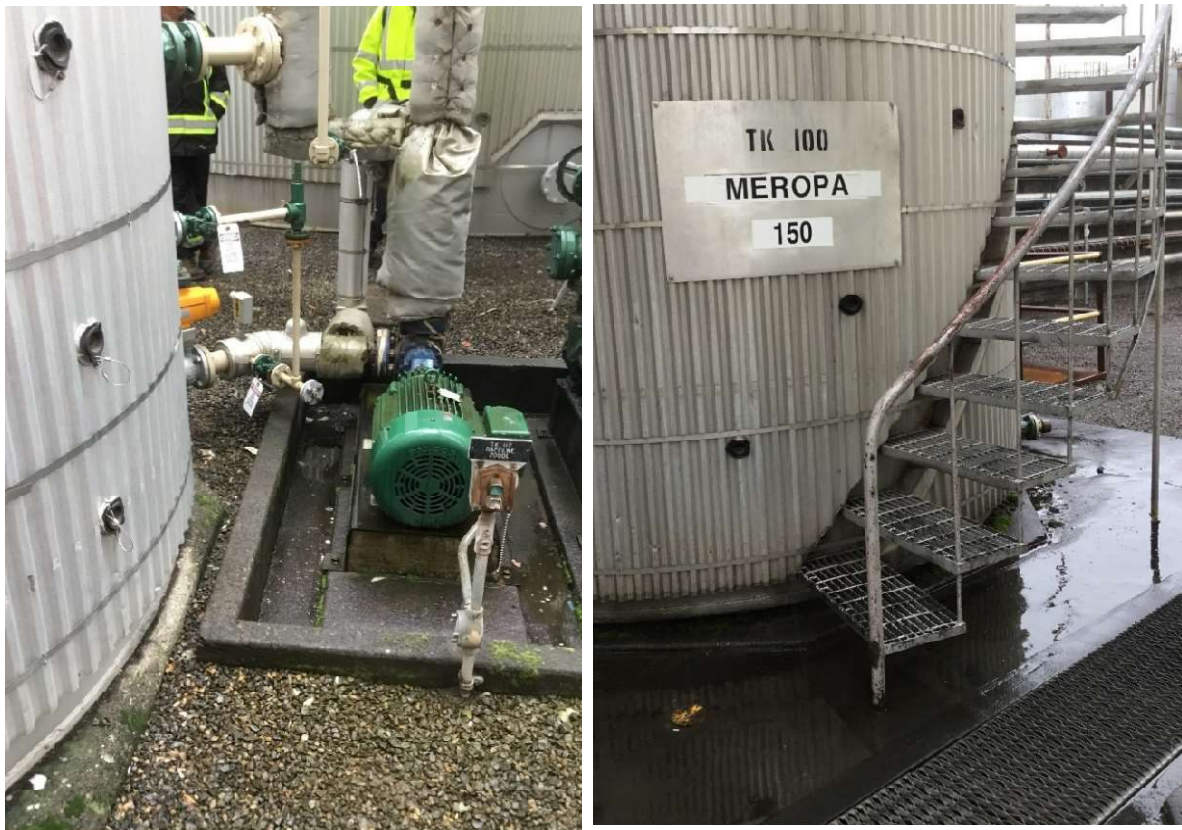
Figure E-1: Example Over-Constrained Conditions Left: Short pipe run to anchored pump at Tank 117 Right: Anchored stair handrail at Tank 100
