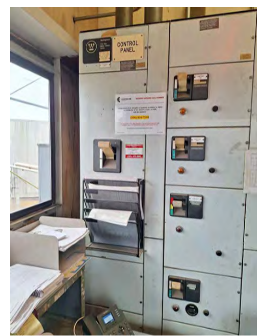
PHOTO #2 - CONTROL PANEL
