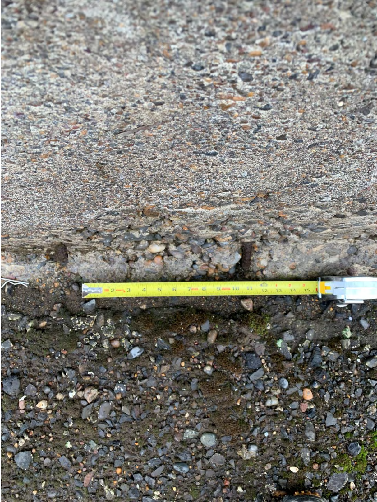
Photo 6 – Concrete Degradation at 6.5-foot Concrete Cantilever Wall
