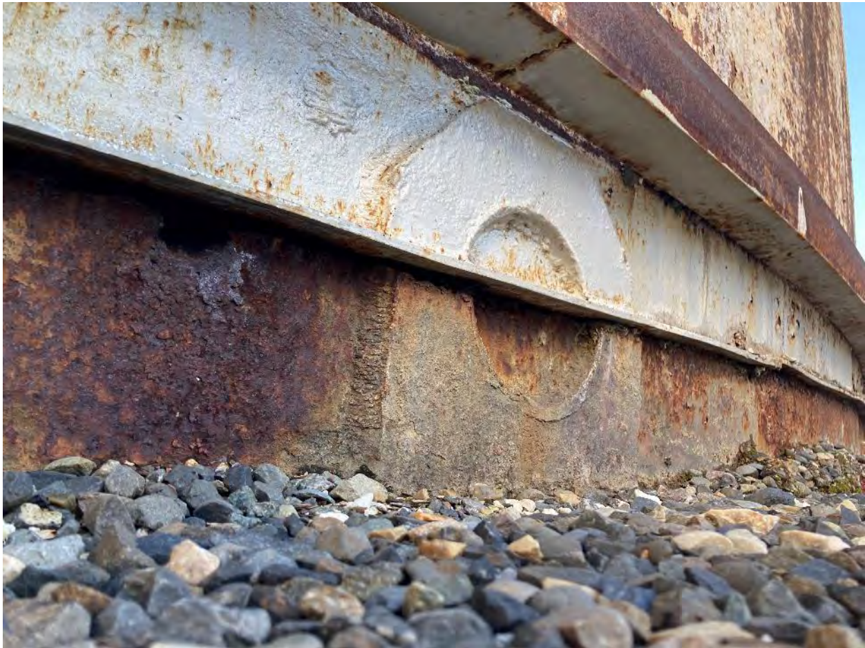
Figure 10. Closeup of Tank 127 non-code tombstone repad.
