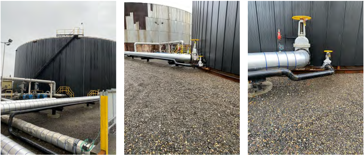
(a) (b) (c) Figure 13. Tank 130 (black tank) and the attached piping system. (a) The piping system attached to Tank 130 with supports under the pipes. (b) A side view of the piping system of Tank 130. (c) A closer view of Tank 130 with attached piping and support.
