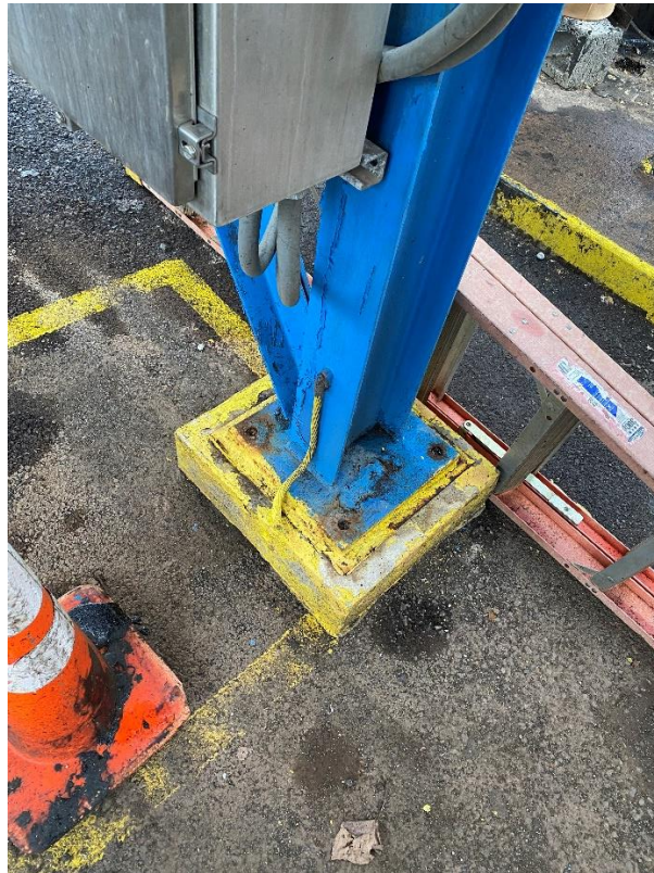
Picture 8. Anchorage not observed at pipe base of Process Area pipe rack.
