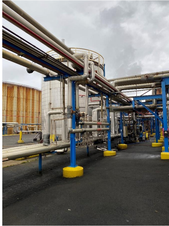
Picture 1. Typical view of Process area.
