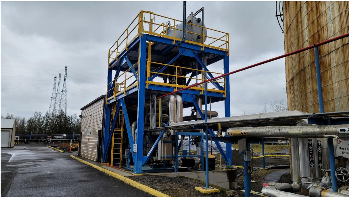
Picture 10. View of hot oil heater building and platform.
