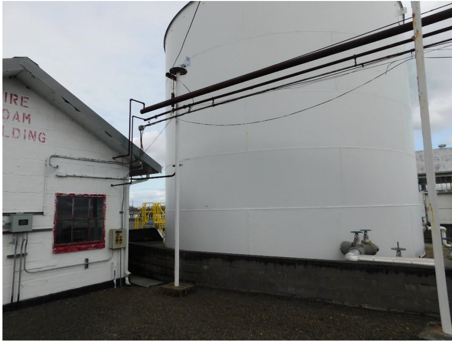
Picture 7. View of slender pipe support at Area 02.
