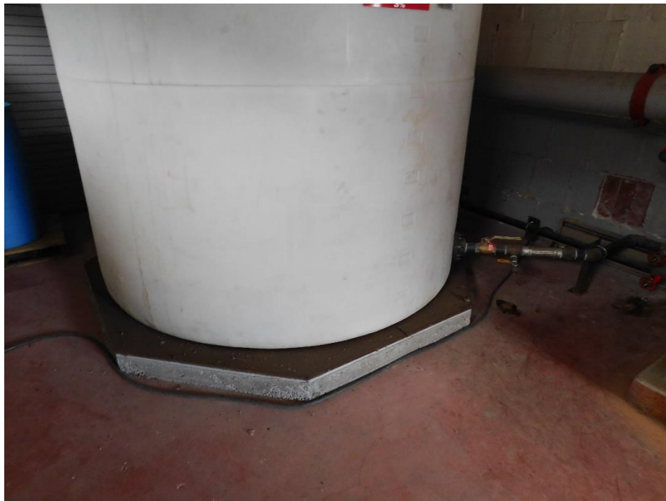
Picture 10. Unanchored foam fire tank at Area 02.
