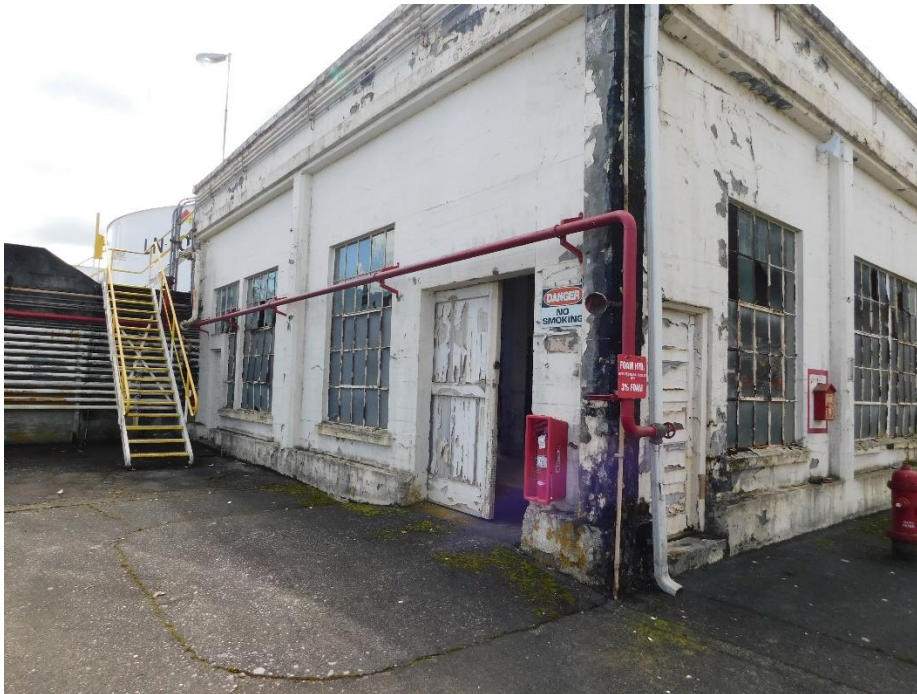
Picture 2. Foam fire pipe supported at Warehouse D.
