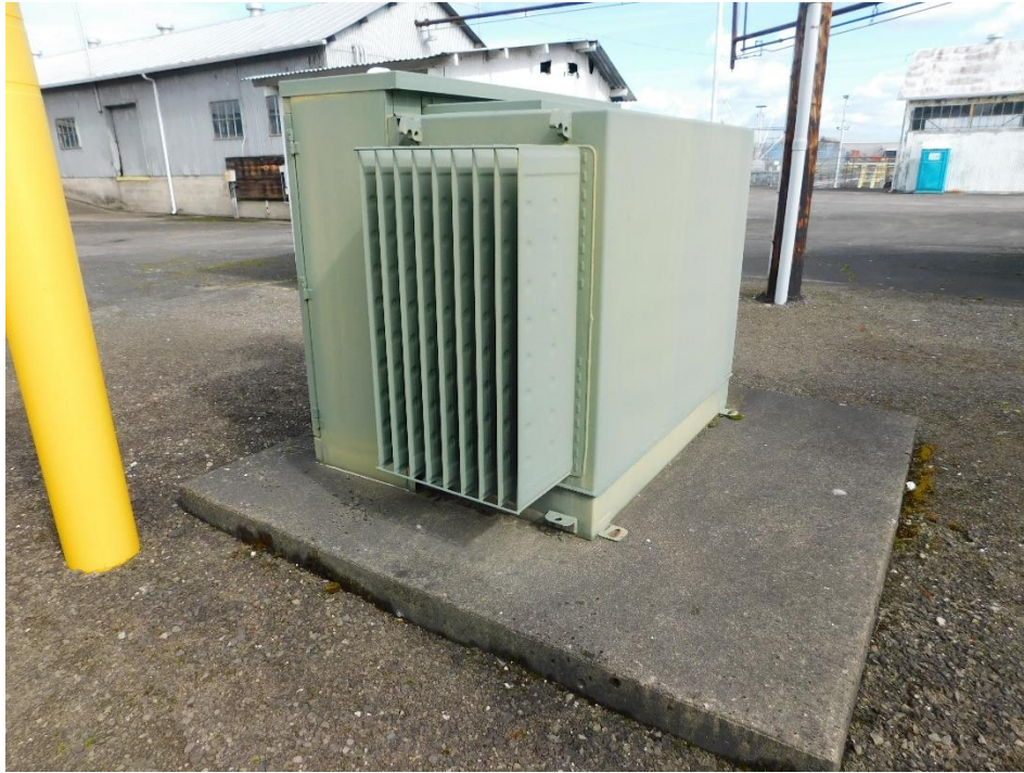
Picture 11. Unanchored electrical transformer at Area 02.
