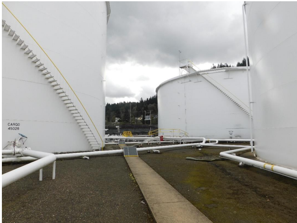
Picture 14. Typical view of tank farm and pipe supports at Area 03.
