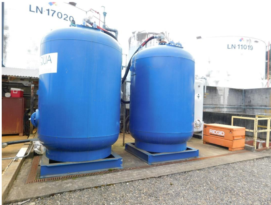
Picture 12. Unanchored water tanks at Area 02.
