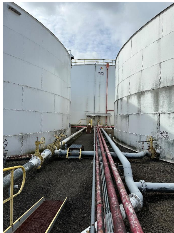
Picture 6. Tank farm and typical pipe supports at Area 02.
