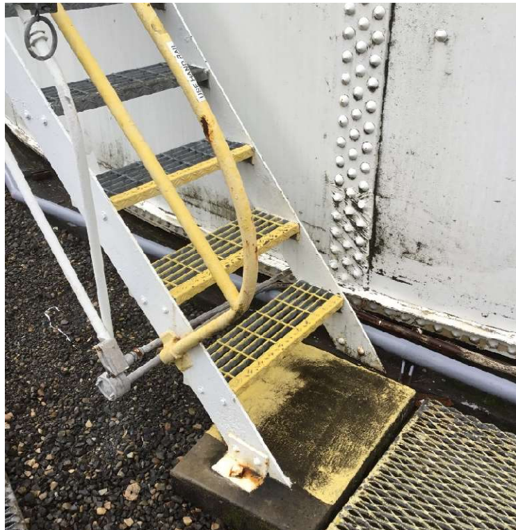
Figure 7-1: Typical Stair Anchorage at South Tank Farm
