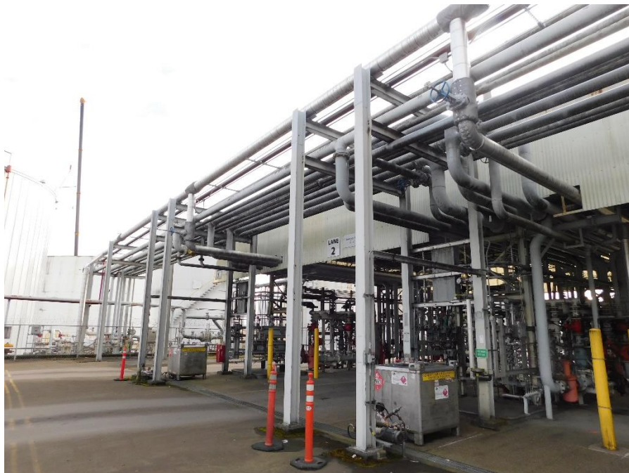
Picture 6. Pipe bridge adjacent to truck loading rack at North Yard.
