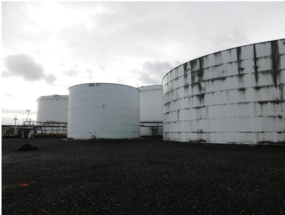
Picture 14. Typical view of tank farm at South Yard.
