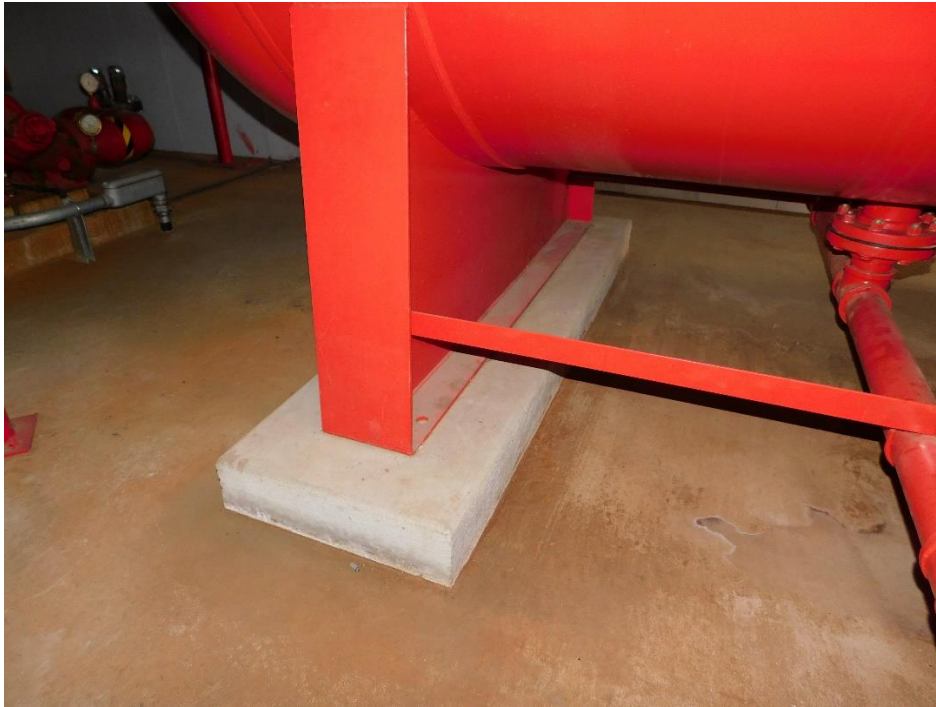
Picture 11. Unanchored gas foam tank at North Yard.
