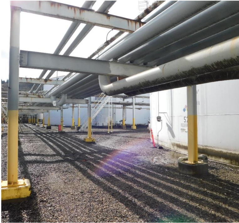
Picture 15. View of typical pipe support type at South Yard.
