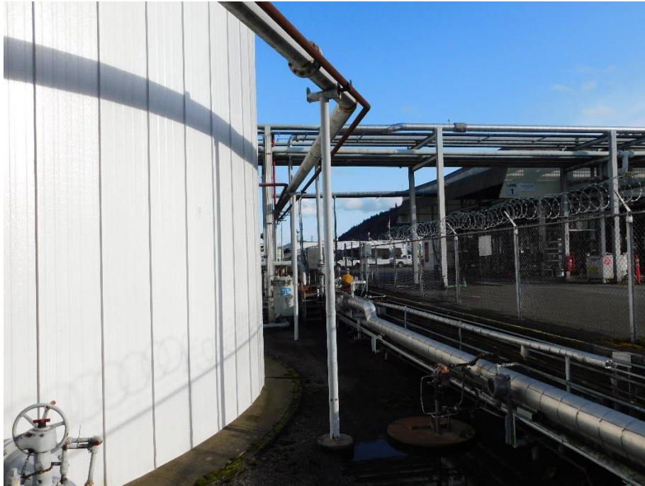
Picture 3. Tall slender pipe support at North Yard.
