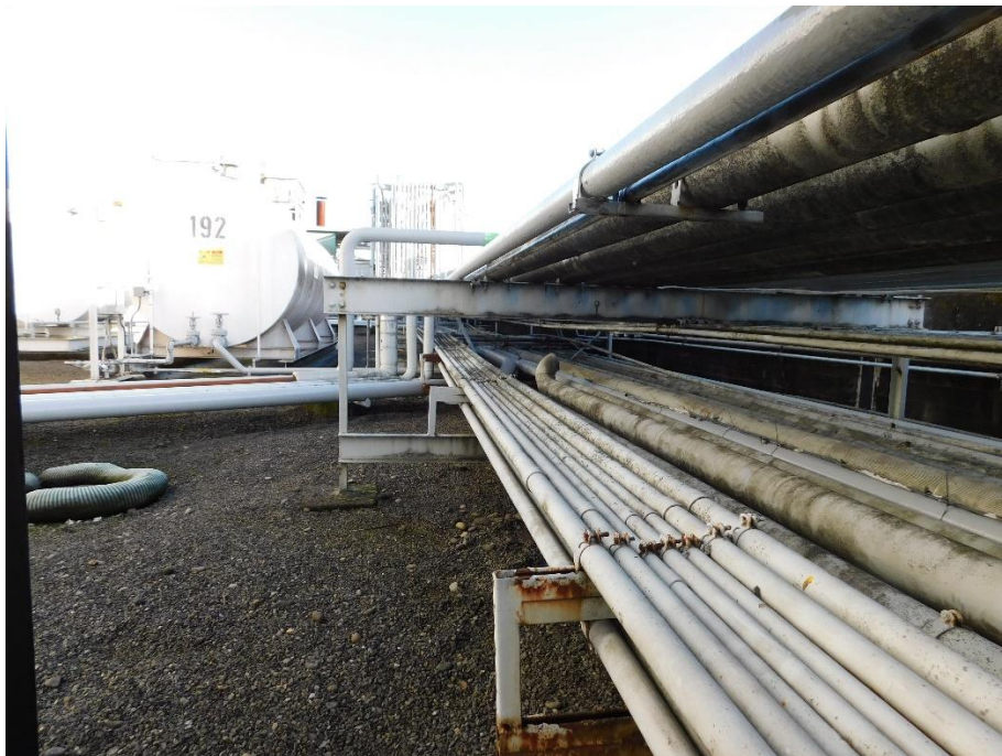
Picture 4. Multiple pipes supported by slender channel framing at North Yard.
