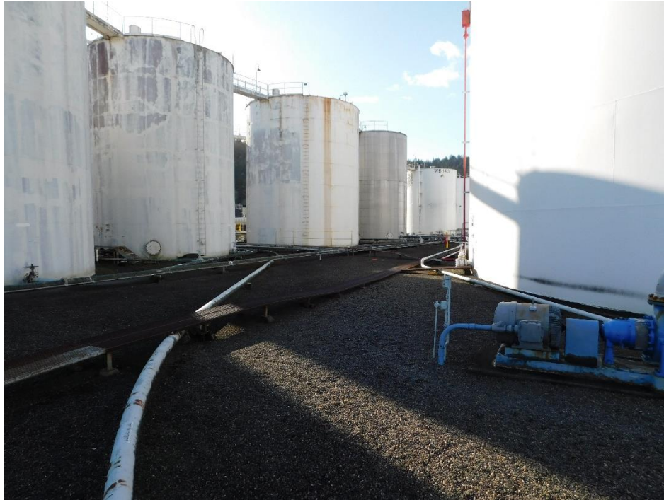
Picture 1. Typical view of North Yard tank farm.
