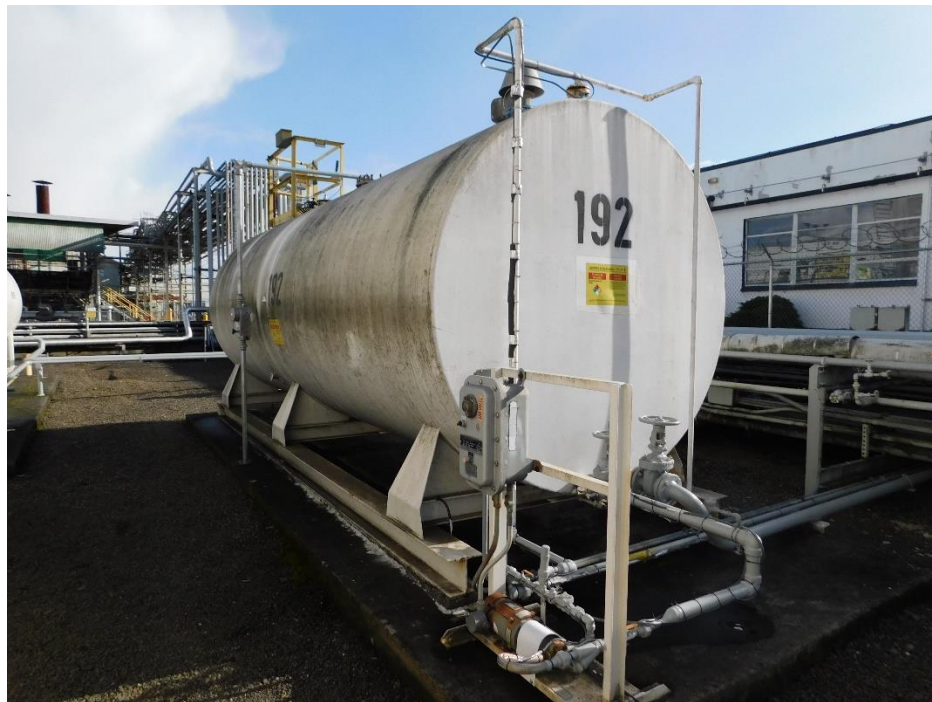
Picture 10. Typical view of unanchored additive tank at North Yard.
