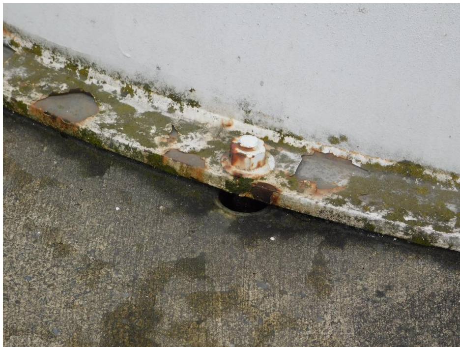
Picture 12. Typical view of North Yard vapor recovery unit anchorage in hole, no epoxy observed.
