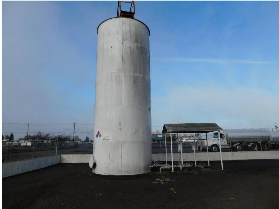
Picture 11. Unanchored vertical additive tank at South Yard.
