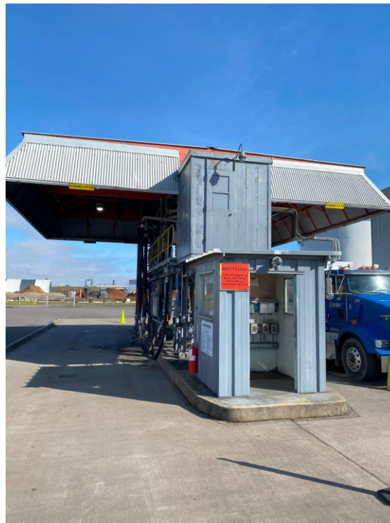
Picture 2. View of typical truck loading rack.
