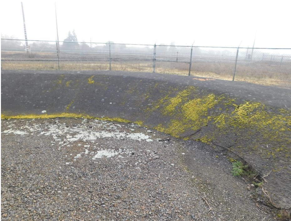
Picture 6. Typical view of gravel berm containment.
