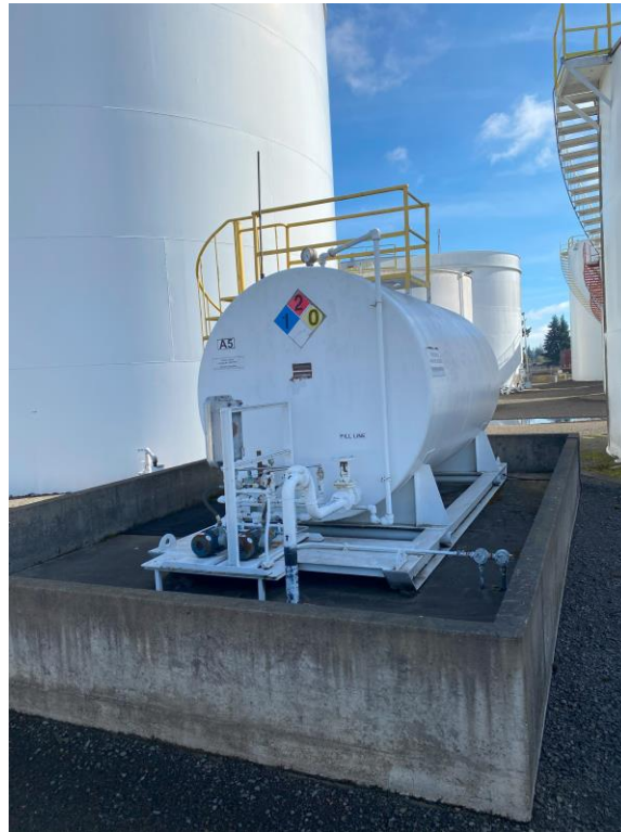
Picture 7. Typical view of unanchored additive tank.
