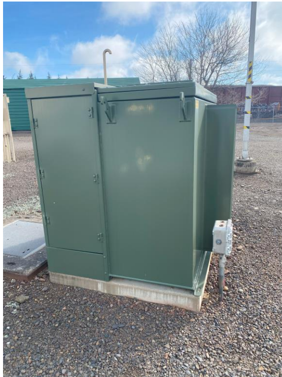
Picture 12. Unanchored electrical transformer at South Yard.
