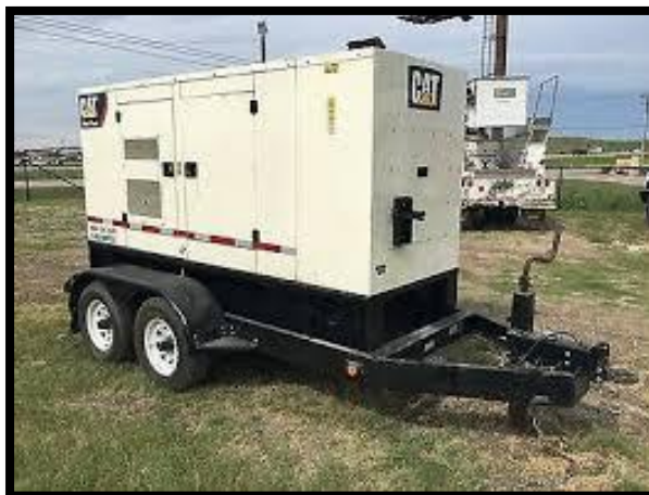
FIGURE 1 EMERGENCY GENERATOR FOR THE WELL FIELD
