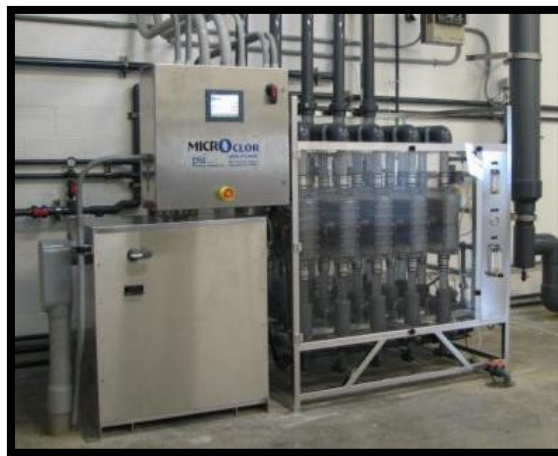
FIGURE 2 PROPOSED WATER TREATMENT PLANT SODIUM HYPOCHLORITE GENERATOR
