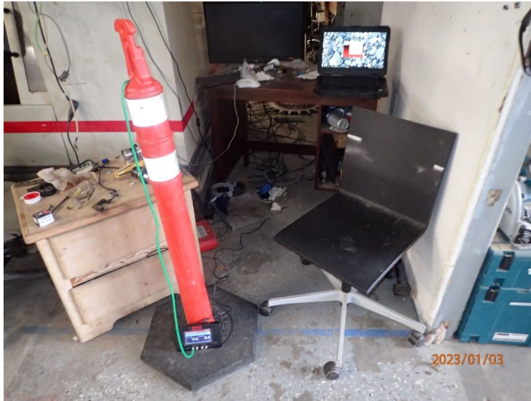
TEC DG-1000 pressure gauge deployed to monitor differential sub-slab pressure at CT14 (outside removal action area) vs. indoor air.
