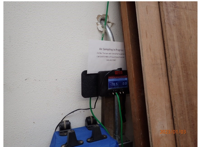
TEC DG-1000 pressure gauge deployed to monitor differential indoor versus outdoor pressures at the west end of the NE warehouse.
