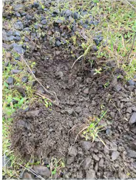
Photo 6 - Closeup view of the gravel layer at the northern portion of the grass field area. A black filter fabric was observed beneath the gravel layer (not yet exposed in the photo above). (12/14/2023)
