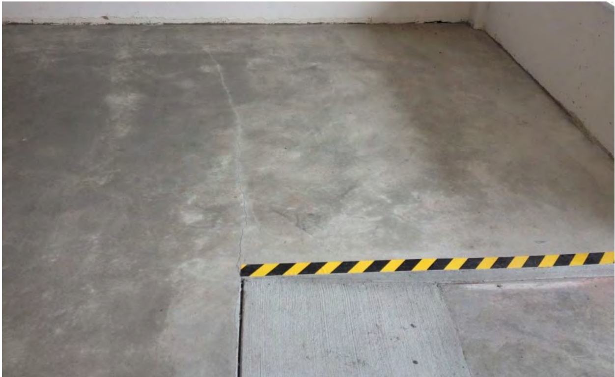
Photograph 14 – As the concrete continued to cure, small cracks formed originating at the corners of the access ramp. These cracks are cosmetic only and do not affect the vapor barrier below.
