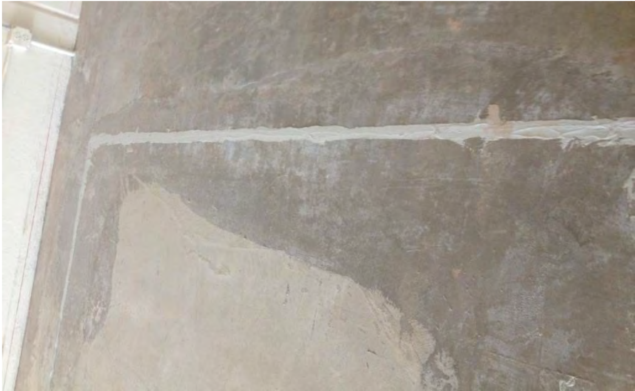
Photograph 2 – Cleaned and sealed cracks around the 2007 IRM excavation.
