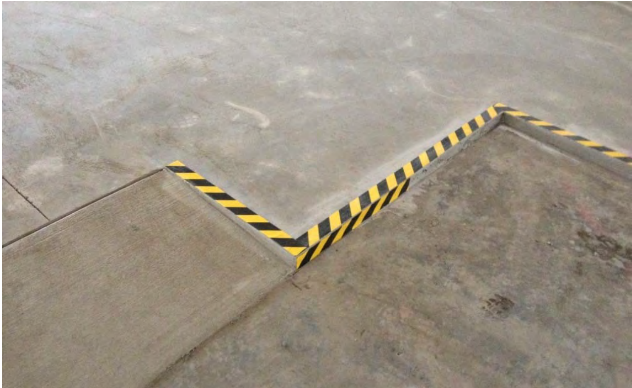
Photograph 13 – Access ramp after curing with caution tape marking trip hazards.
