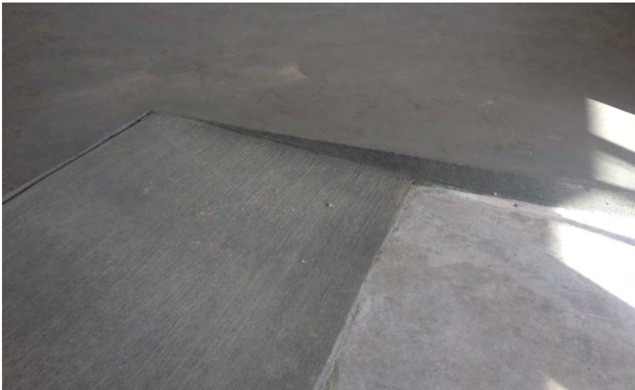
Photograph 12 – One of the access ramps after the formwork was removed. Note the ramp is textured while the top of the slab is smooth.
