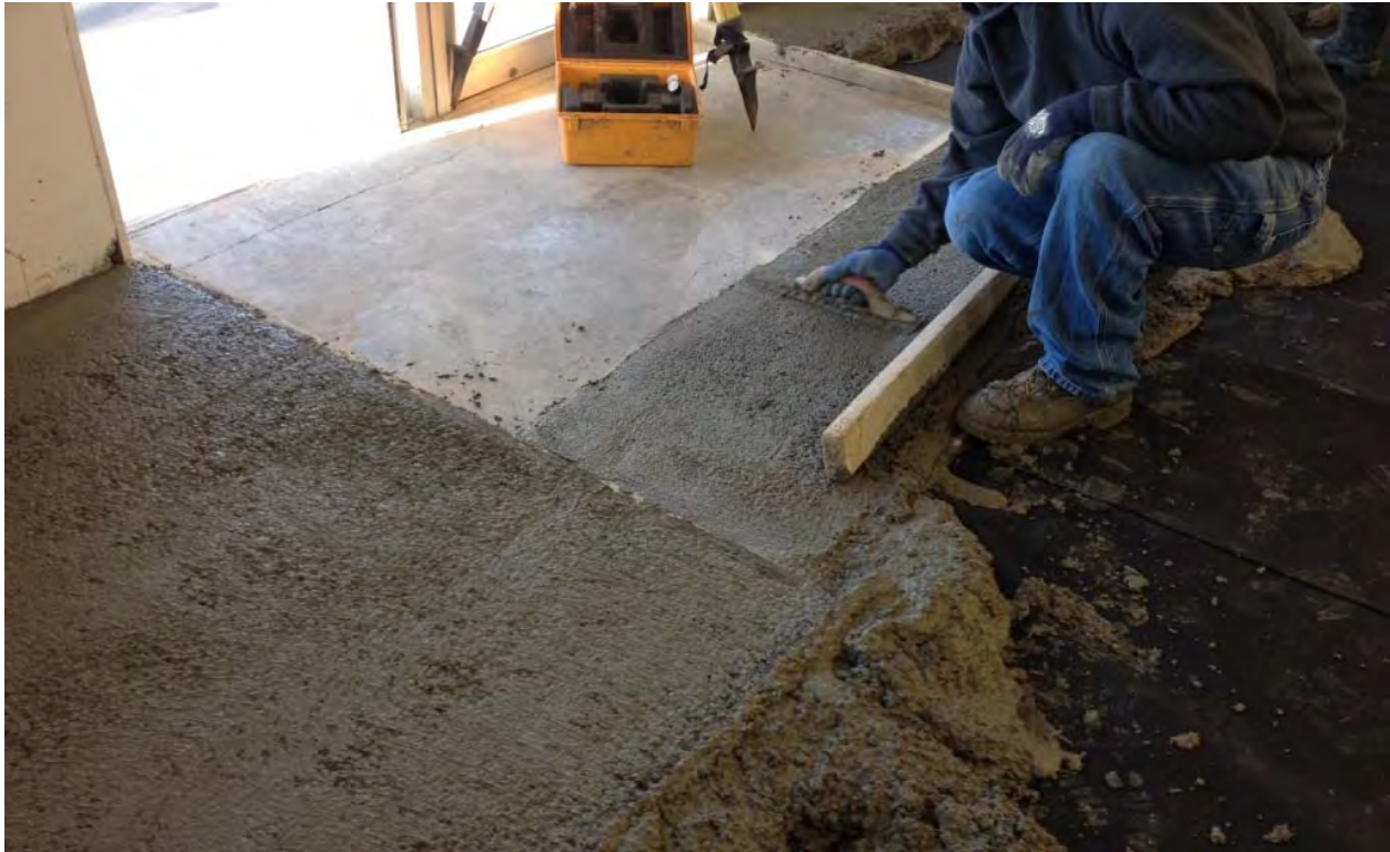
Photograph 9 – Concrete slab progress. Photograph shows an access ramp beginning to take shape.
