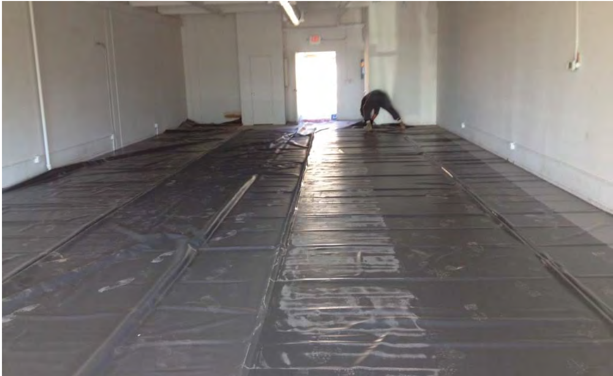
Photograph 5 – PVC liner is laid out in one piece, the crew is adjusting the liner and will cut the sections that do not require the vapor barrier.
