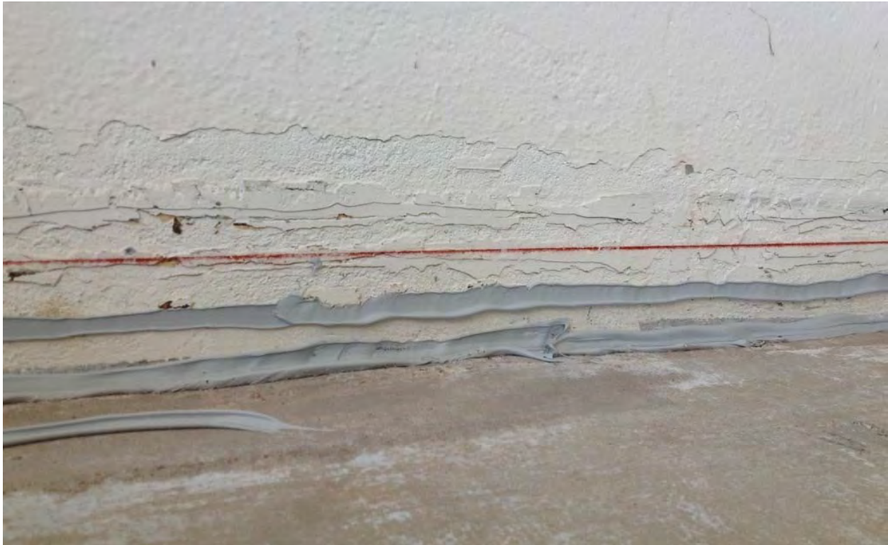
Photograph 3 – Two inches above the existing slab is marked by the red line. The PVC liner is ready to be installed with the edge of the concrete slab sealed as well as on the wall where the PVC liner will rest.
