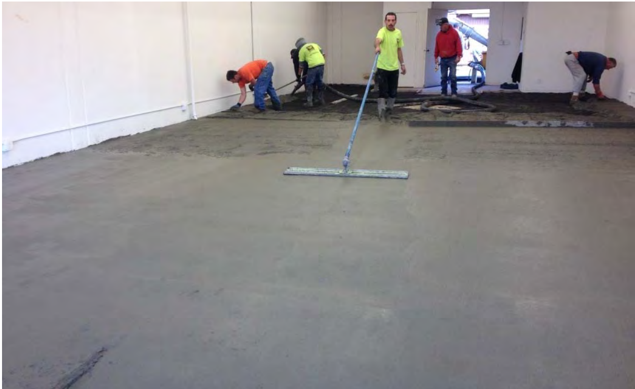
Photograph 10 – Concrete was smoothed as the crew worked towards the back of the retail space.
