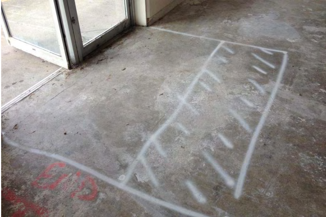
Photograph 5 – Photograph of the front doorway. The white line delineates the boundary of the vapor barrier. The vapor barrier will not go up to the doorway. The hatch marked region shows where a small ramp will be installed.
