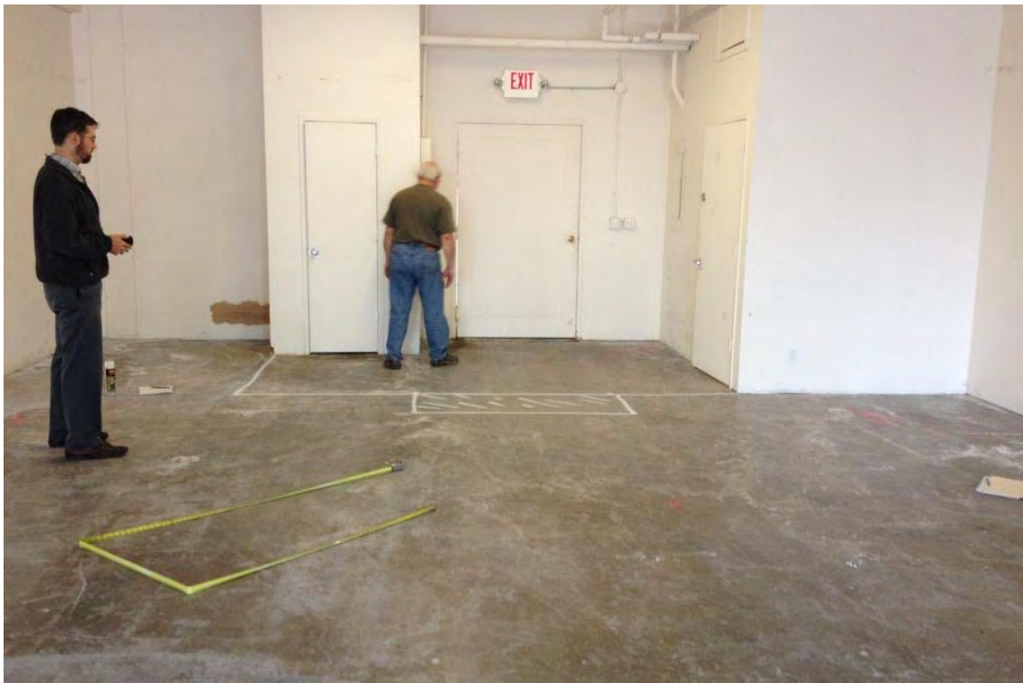
Photograph 6 - Photograph of the back doorway. The white line delineates the boundary of the vapor barrier. The vapor barrier will not go up to the doorway. The hatch marked region shows where a small ramp will be installed.
