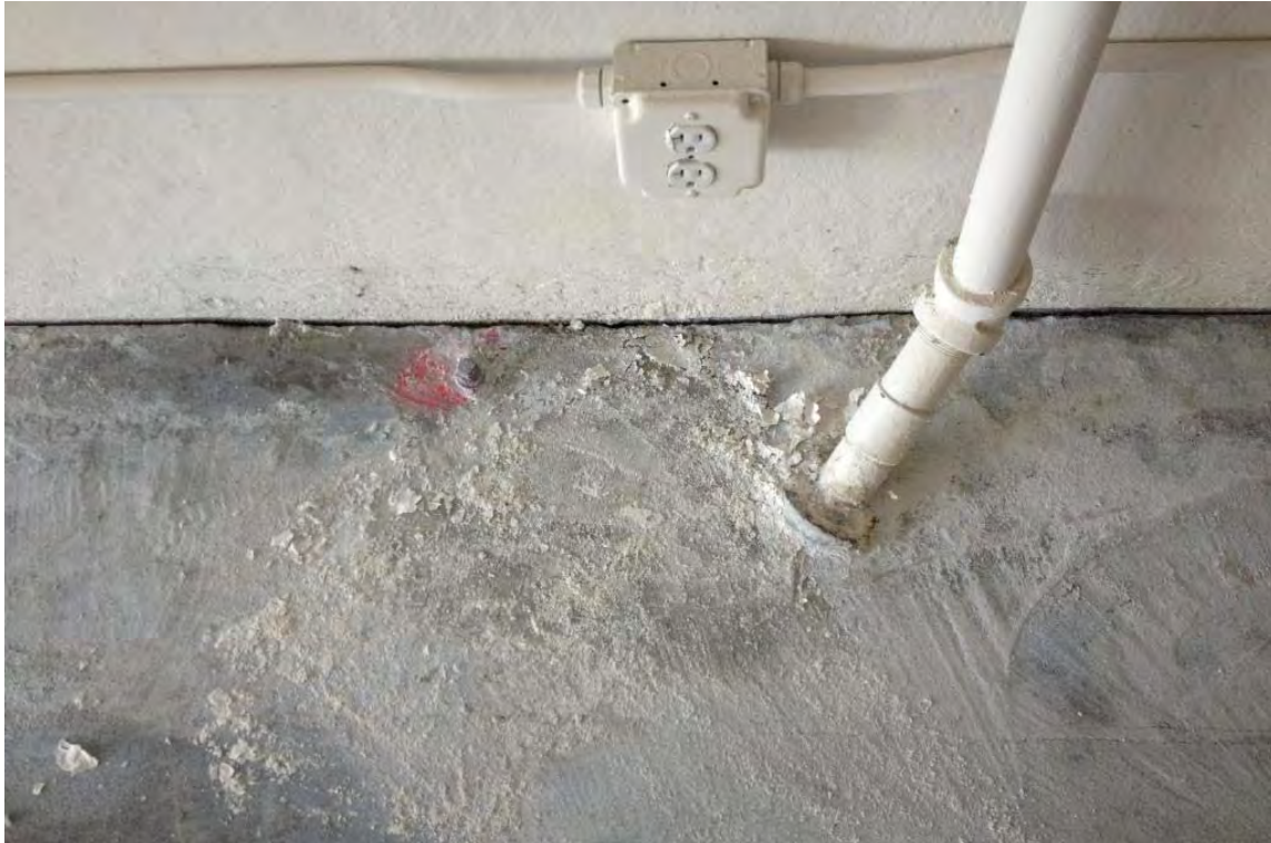
Photograph 4 – Close up image of typical gap between the current floor slab and the wall to be sealed prior to vapor barrier installation. Photograph shows a utility pipe that will require to be sealed during vapor barrier installation. Towards the center of the photograph (next to small red paint) is an existing power conduit which is currently capped. This will need to be extended two inches and capped flush with the new concrete slab.
