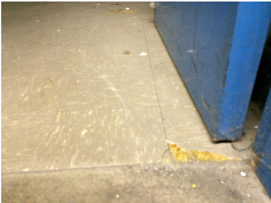
VIEW OF THE ASBESTOS-CONTAINING FLOOR TILE LOCATED WITHIN THE SHOP OFFICE.
