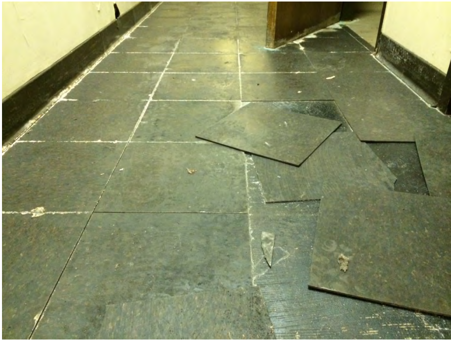
VIEW OF THE ASBESTOS-CONTAINING FLOOR TILE AND MASTIC LOCATED IN THE UPSTAIRS OFFICE.
