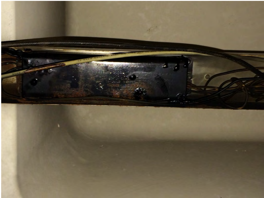
PCB BALLAST LOCATED IN CENTRAL PORTION OF THE BUILDING.
