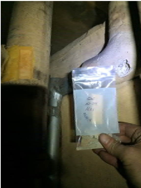
VIEW OF AN ASBESTOS-CONTAINING HARD PIPE FITTING LOCATED IN THE ROOFTOP MECHANICAL ROOM.
