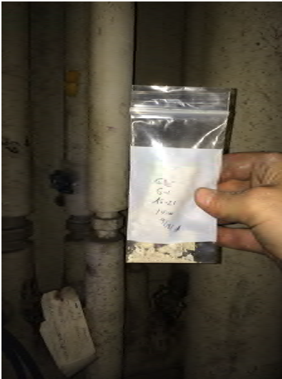
VIEW OF AN ASBESTOS-CONTAINING HARD PIPE FITTING LOCATED IN THE BOILER ROOM.
