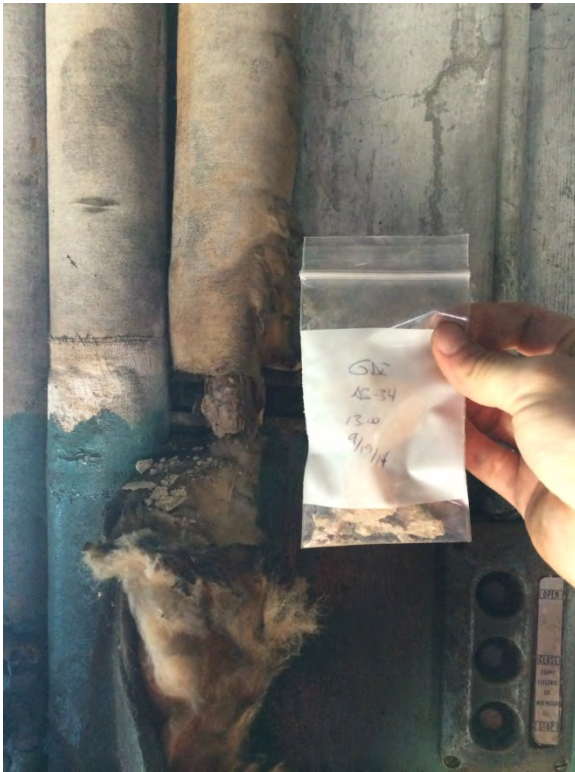
VIEW OF AN ASBESTOS-CONTAINING HARD FITTING LOCATED IN THE EASTERN SHOP AREA.
