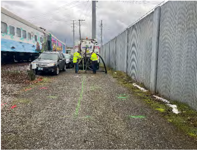
Holt clearing boring location via an air knife. Utility marks shown in the background.
