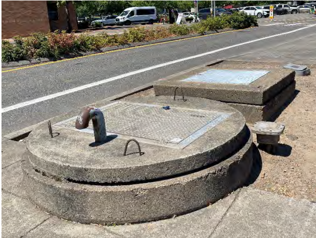
Water infrastructure in front of OMSI.
