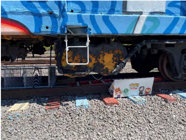
Grey water tank under stationary railcar with unknown insulation.
