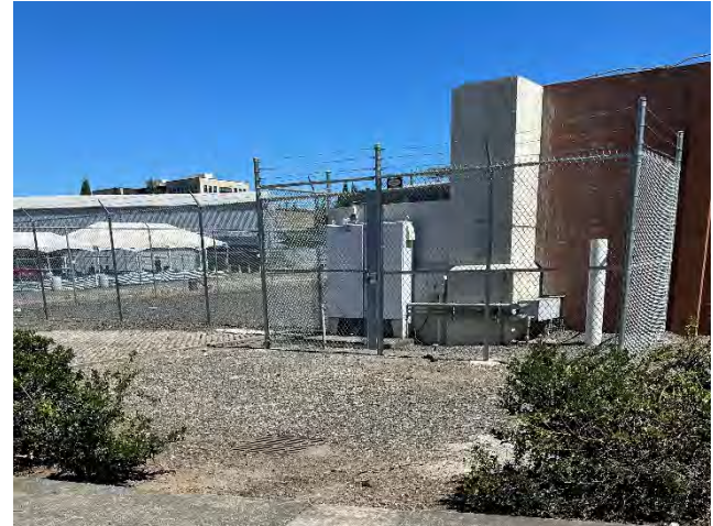
Electrical utilities located on PG&E property.
