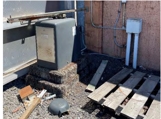
Gate motor for PG&E's gate.
