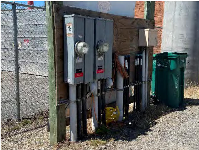
Electrical panel for the stationary railcars.
