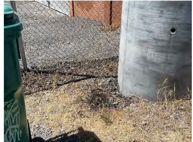
De minimis surface staining.
