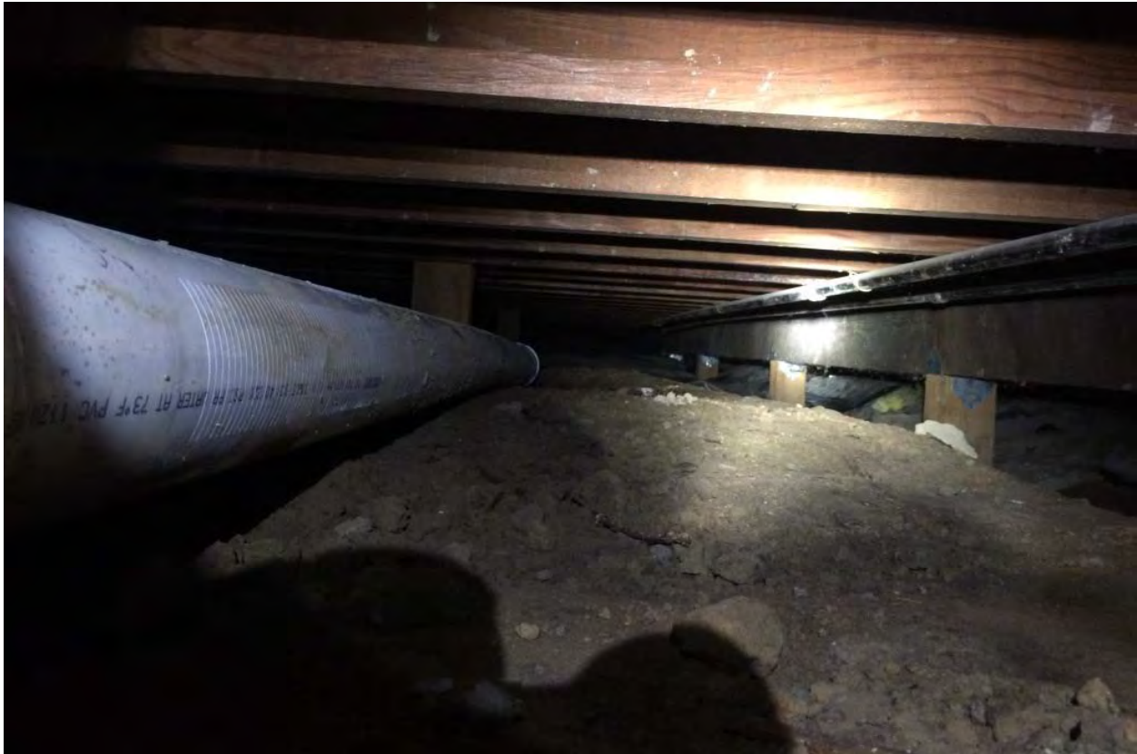
Photograph 11 – The crawlspace with the slotted PVC soil gas collection pipe to the left. The building support piers can be seen on the right.
