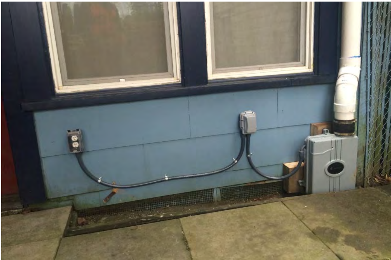
Photograph 12 – The in-line ventilation fan secured to the north side of the building on the right. The fan is wired to the outlet on the left and fitted with a power switch (center). The exhaust stack can also be viewed exiting the fan housing vertically. Photograph taken facing south.
