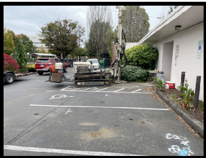
Photograph 3: Location of Phase II ESA boring P4. The spray painted white "T's" indicate the extent of the former UST excavation fill area. The Subject Property Building is on the right side of the photograph.
