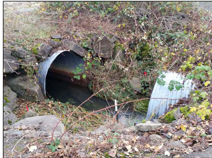
Photo C. Overview of Unknown Reach (between 1 and 2), Bear Creek. Photo by E. Dulin on November 23, 2015.
