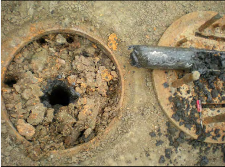
PHOTO 1 Catch basin prior to cleaning.
