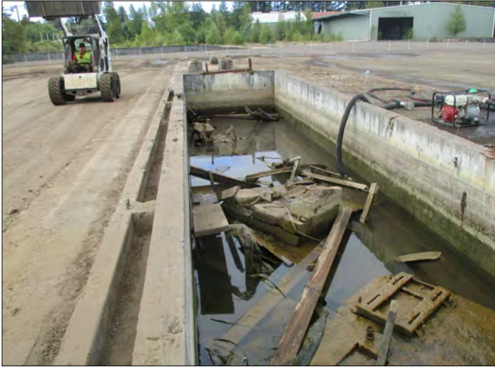
PHOTO 7 Former Dip Tank #2 concrete containment vault debris.
