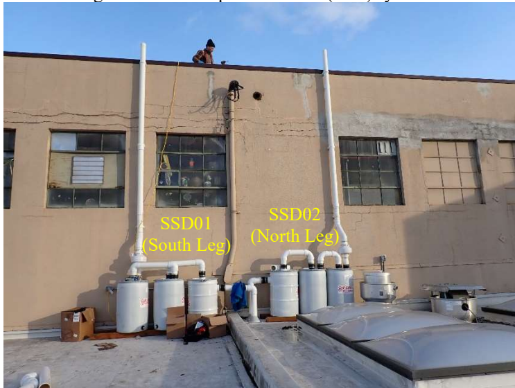
SSD system with one inline fan and three GAC units per vent.
