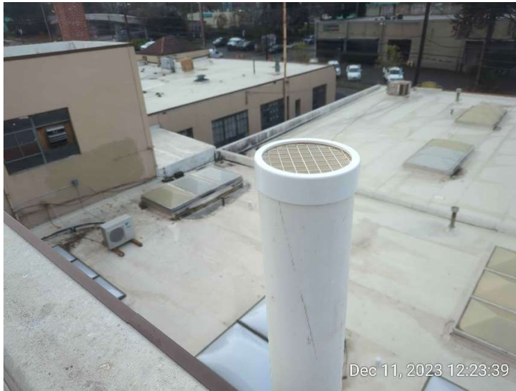
Critter-guards on vent risers.
