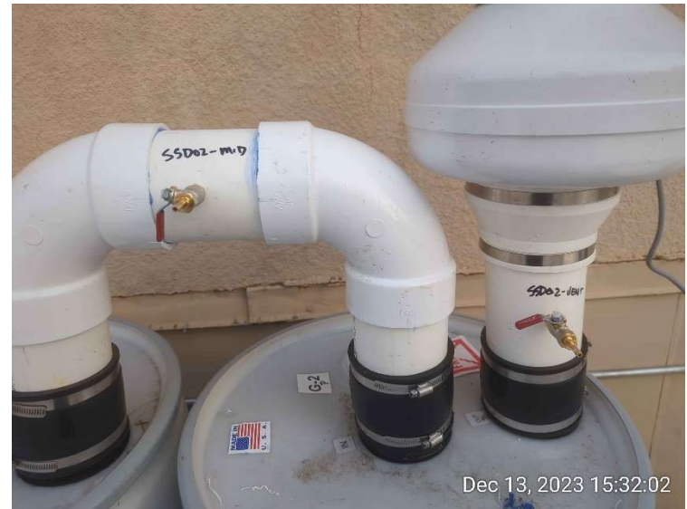
Mid-GAC and vent sample ports.
