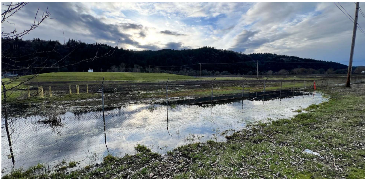
Photo 2: View of stormwater ponding in the low field looking West from NW Front Ave.
