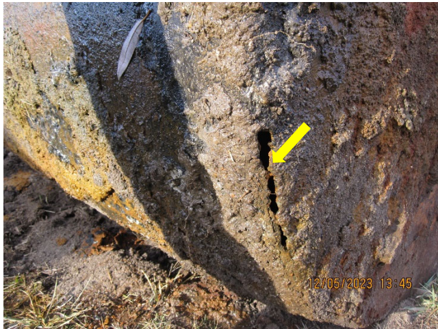
Photo 9: Looking at bottom of UST. Arrow points to corroded seam.
