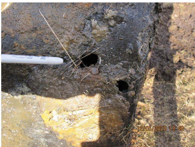
Photo 11: Closeup of larger holes in bottom of UST; marker pen for scale.
