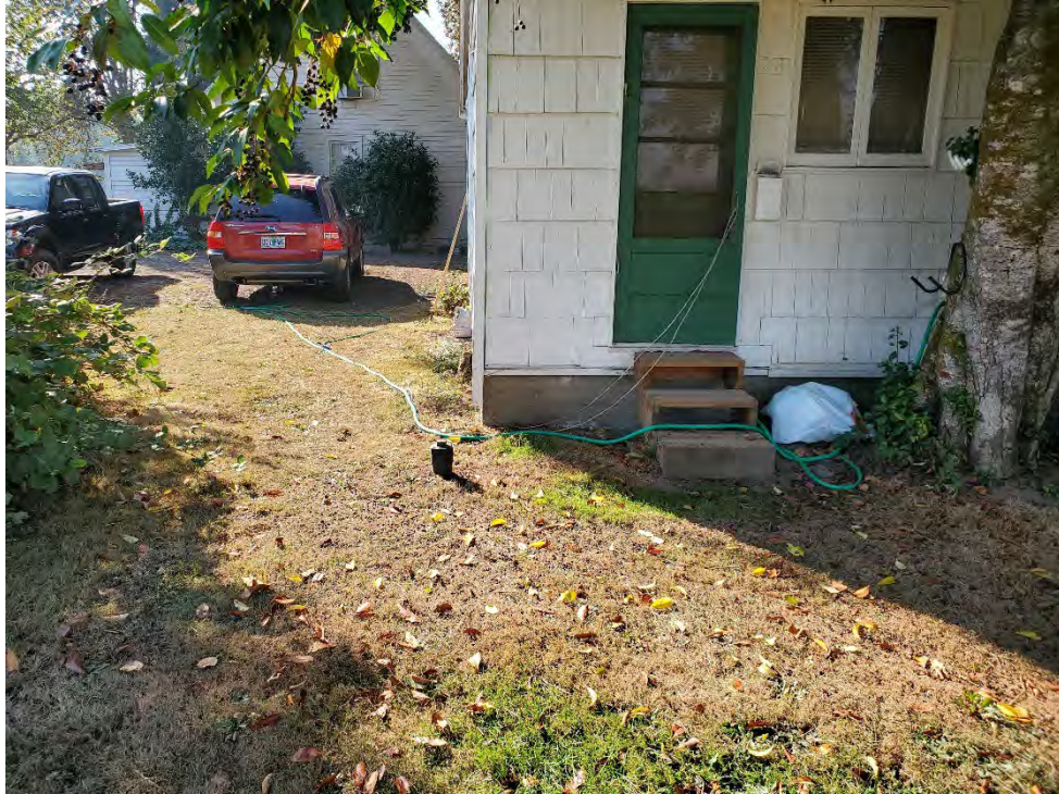
View of apparent sewer cleanout pipe at northeast corner of duplex.
