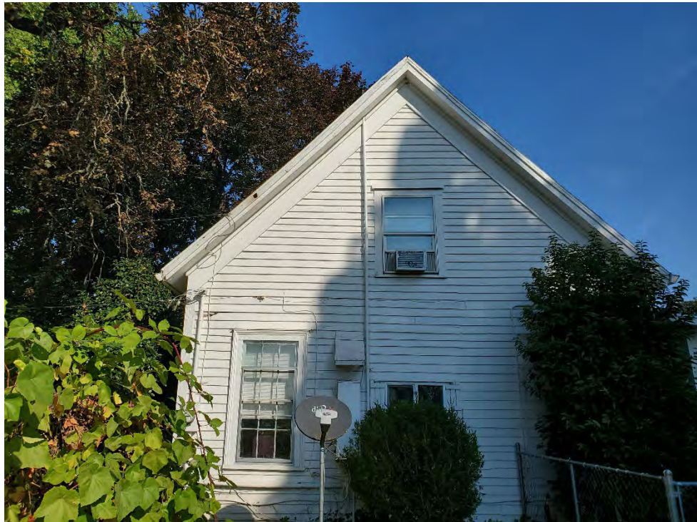
View of pipe attached to outside and protruding through roof on south side of farmhouse.
