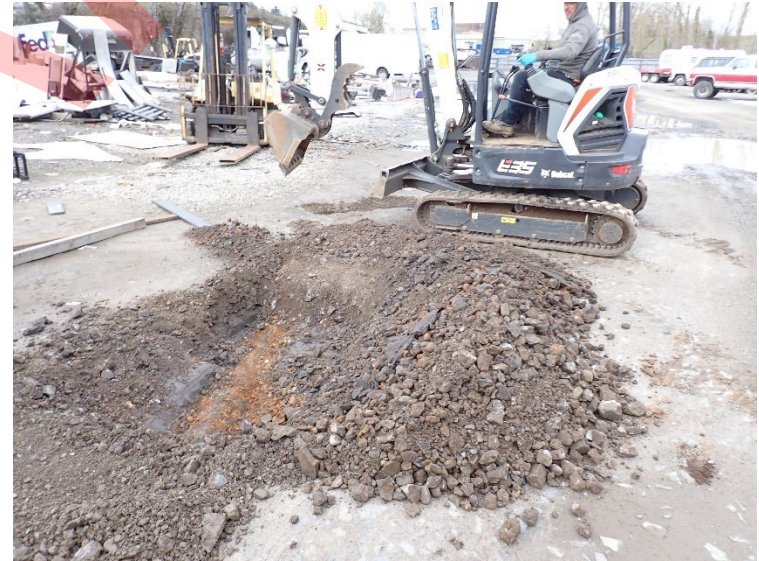
Magnetic anomaly MA20 was excavated to reveal an 11-foot-long, open ended, section of a steel pipe buried horizontally.
