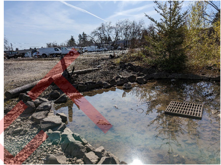
Ponded area and grated drain at the west side of the property.
