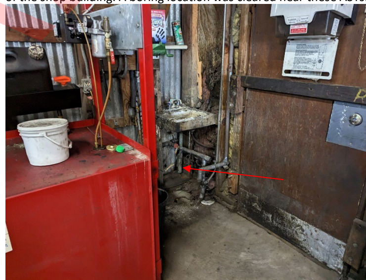
The hose drain for the shop sink was observed that protruded through the wall of the shop building.
