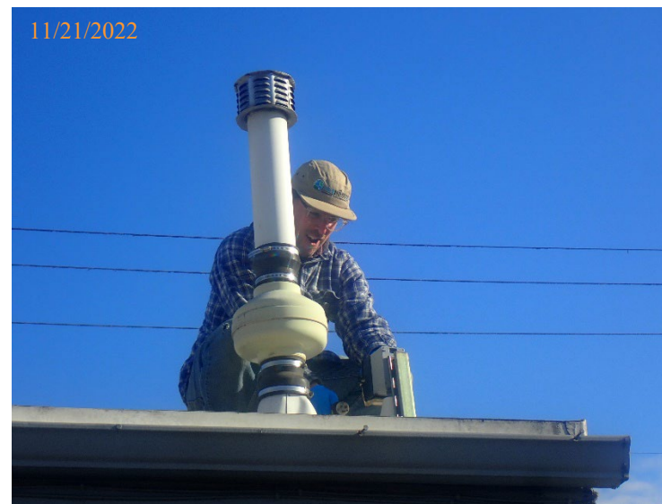
Setting the SSD in passive mode, i.e., powering off the radon fan, after collecting a vapor sample from the vent riser.
