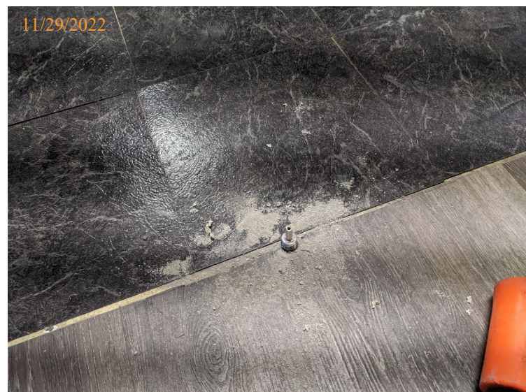
Vapor Pin for SUB07 in space 1240.
