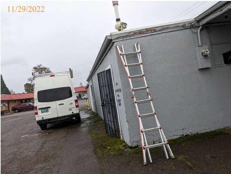
The inline fan was powered on for 1 minute to purge lines, and then turned off to sample the SSD vent on 11/29/2022.
