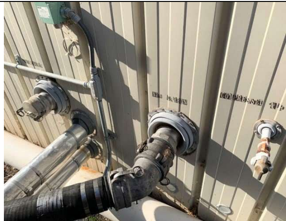
New carbon entering the building
