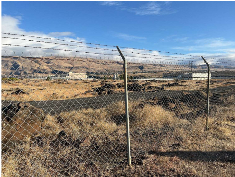
Evidence of burrowing under CERCLA landfill fence
