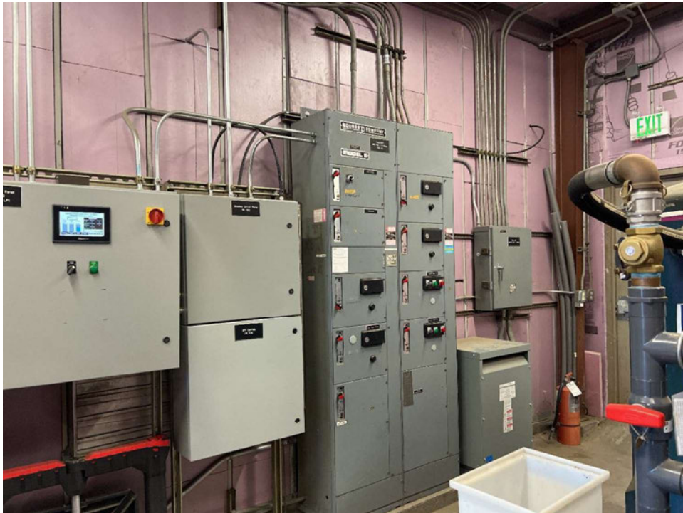
Treatment plant main control panel
