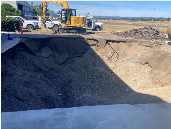
Photo #1 Tank nest following removal of USTs from subsurface – looking north-northeast with Teufel Hangar to left.
