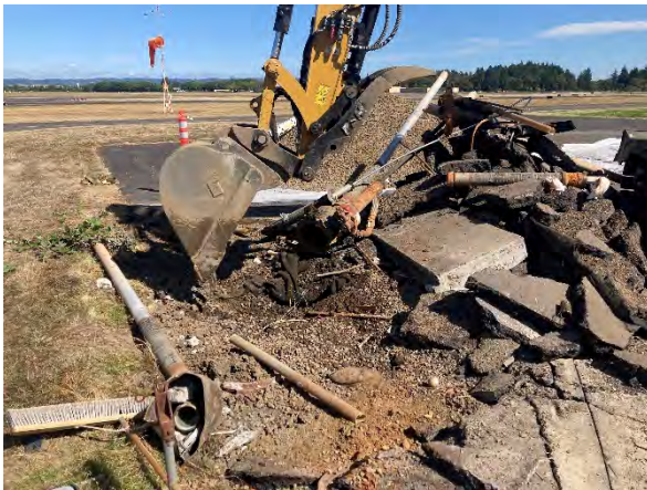
Photo #9 Start of excavation at former fueling area on northeast portion of property.
