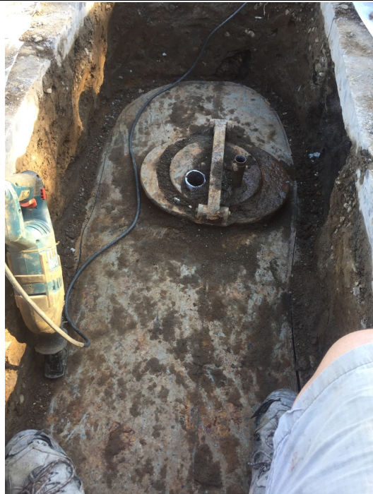
SSES removed the concrete located above the UST and dug to the top of the UST. The overburden soil was placed on plastic sheeting for disposal. SSES personnel inerted the UST and cut it open.
