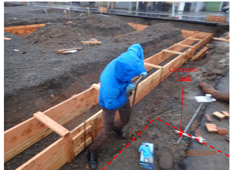
Using a stainless-steel hand auger to advance boring B13 in the footing excavation on the NE side of an abandoned concrete flow-through tank.
