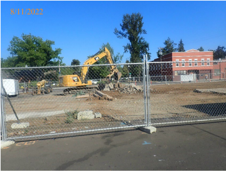
The site following building demolition. View NW toward N 1 st Street from the alley to the SE.
