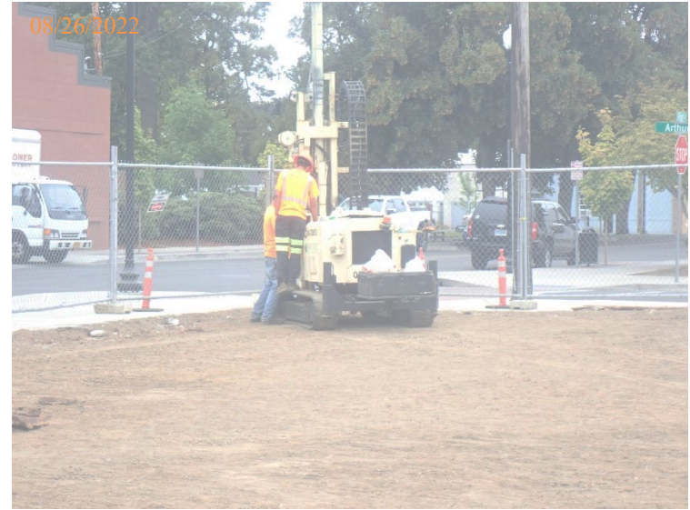
Direct-push drilling rig set up at B01 at the N corner of the property.
