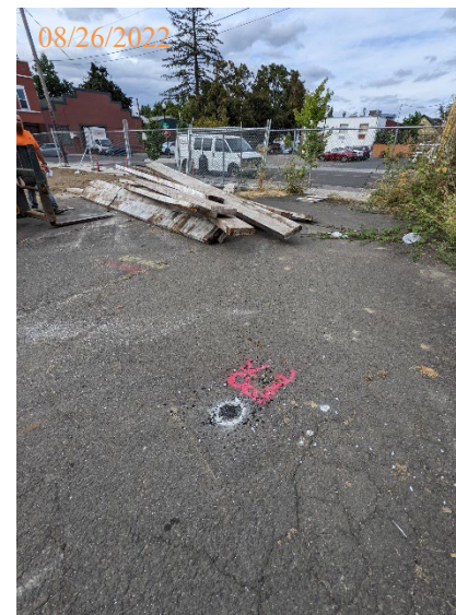
All temporary boreholes were abandoned with bentonite chips and the surface restored to match existing surface.
