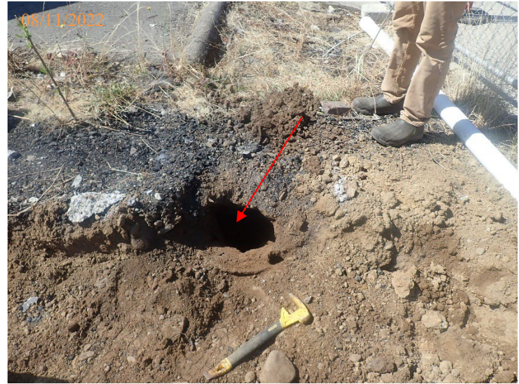
Excavation of MA01 near the NW site corner revealed a deteriorated empty steel drum (on end), which may have been used as a dry well.
