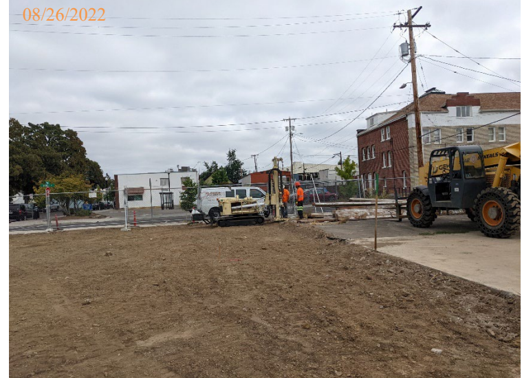
Drill rig set up at B03 at the edge of the former parking area near the E corner of the site.
