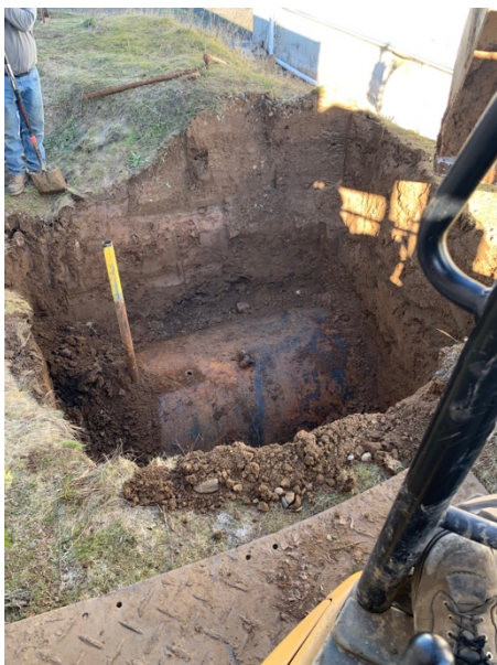
Photo 5. Exposed 1,400-gallon diesel UST.
