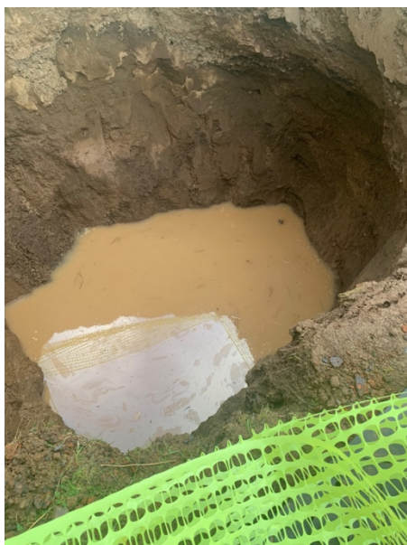
Photo 11. Groundwater in the tank pit.
