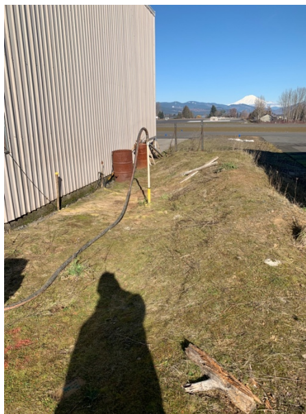
Photo 2. Fill pipe over W end of UST with SSES pump running down pipe. View is to the NNW.
