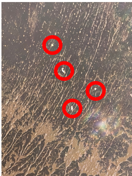
Photo 9. Holes in the UST exterior circled in red.
