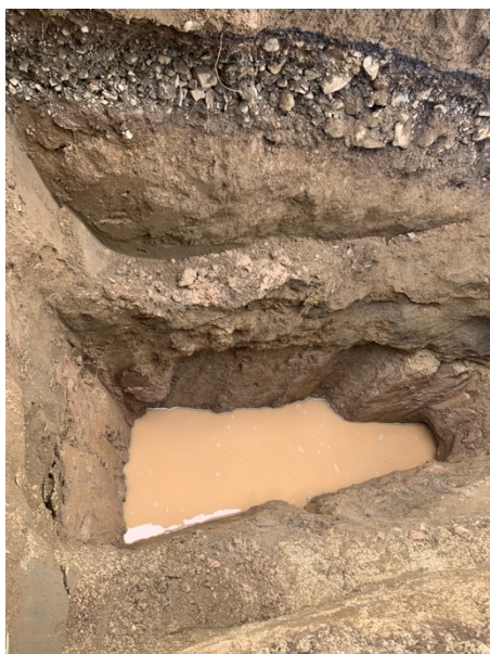
Photo 19. Groundwater recovery trench being recharged by groundwater.
