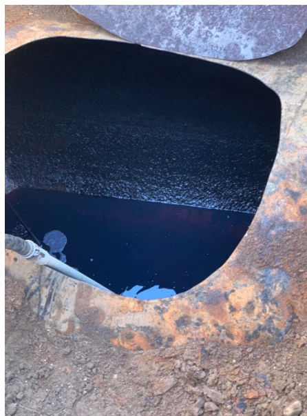
Photo 6. Interior of UST. Approximately 909.6 gallons of fuel was removed.
