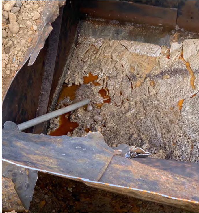
Tank 3 was cut open and found filled with concrete slurry.
