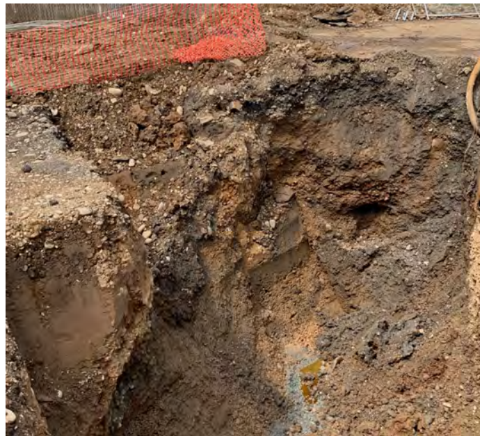
An estimated 100 tons of PCS was removed from the former area of tank 1.
