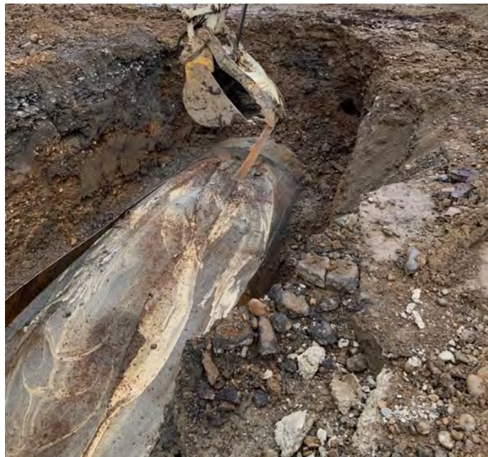
Tank 2 was cut open and found filled with concrete slurry.
