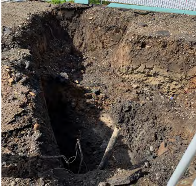
A portion of the top of the tank was exposed and cut open.
