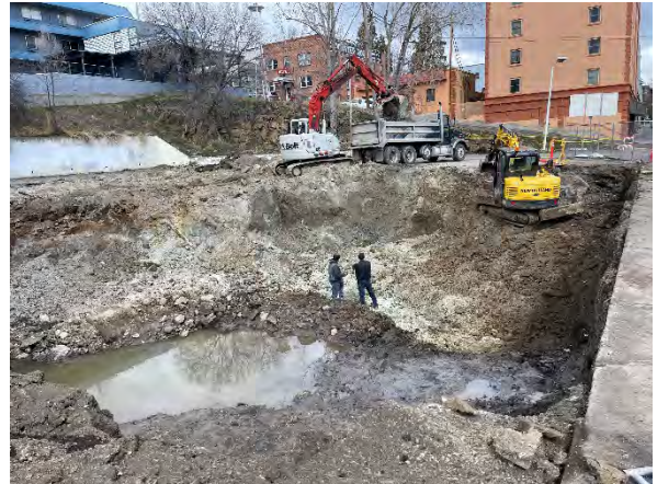
Photo #26 Remedial excavation extended to the north showing former tank nest in foreground.
