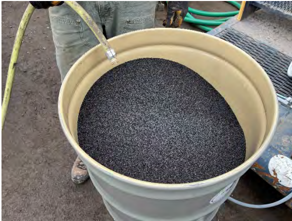
Photo #13 Activated carbon in 55-gallon drum being primed for treatment of water removed from excavation.
