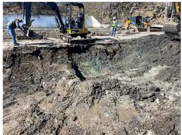
Photo #24 PCS in the vicinity of the west pump island and northwest dispenser.
