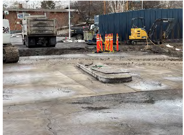
Photo #2 West pump island and fuel dispenser sump with drive lanes on either side.
