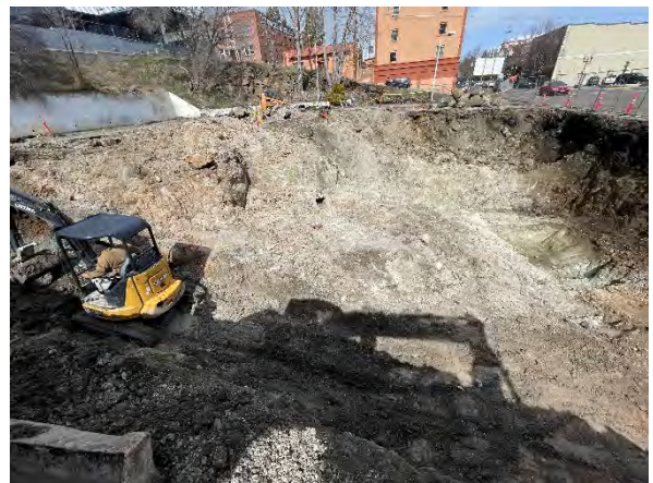
Photo #30 Remedial excavation viewed from south end of former tank nest looking north – excavation remained dry for several days.
