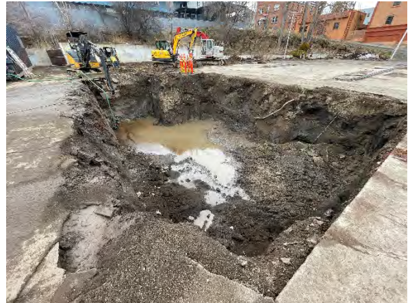
Photo #14 Water in tank nest excavation during pumping.
