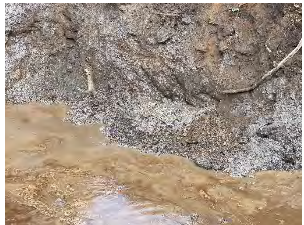
Photo #12 Surface water entering excavation from shallow gravel layer on north tank nest excavation sidewall.
