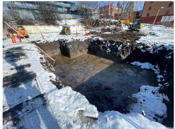
Photo #18 Tank nest excavation filling with additional surface water from recent precipitation and snowmelt.
