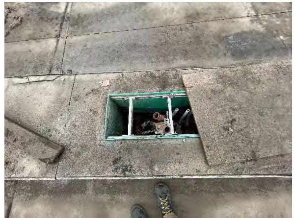
Photo #4 View of product piping and fuel dispenser sump.
