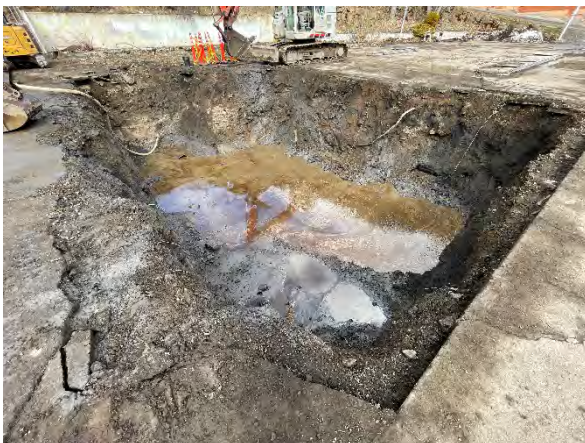
Photo #11 Water in tank nest excavation during pumping.
