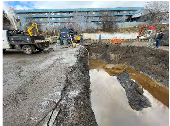
Photo #10 Pondered water remaining in tank nest excavation following UST removal – ES&S setting up pump for removal of water.
