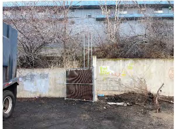
Photo #8 Vent pipes from three gasoline USTs at the Site.
