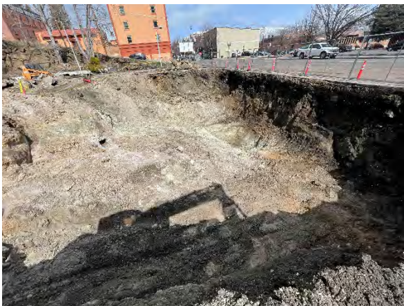
Photo #29 Remedial excavation viewed from south end of former tank nest looking north – excavation remained dry for several days.
