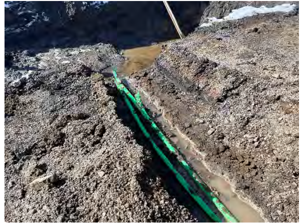
Photo #20 Product piping run from tank nest to first dispenser (southeast dispenser).
