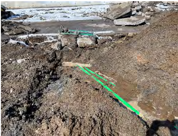
Photo #21 Product piping run from second dispenser (northeast) to third dispenser (northwest).
