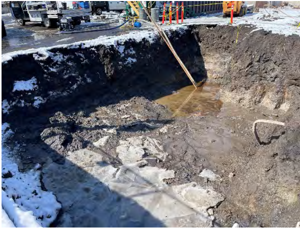
Photo #19 Tank nest excavation after pumping surface water from sump created in southwest corner of excavation.
