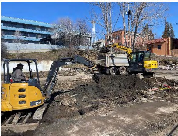
Photo #23 ES&S excavating PCS from north tank nest sidewall to the north in the vicinity of the former western pump island – PCS directly loaded into trucks.
