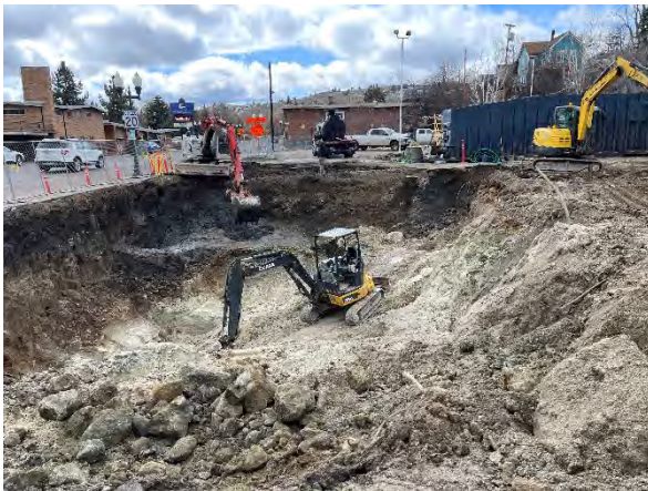
Photo #27 Remedial excavation viewed from the north of the Site – ES&S excavating PCS from tank nest floor (back left of photograph).
