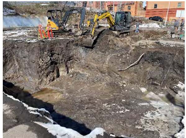
Photo #22 ES&S excavating PCS from north tank nest sidewall to the north in the vicinity of the former western pump island.
