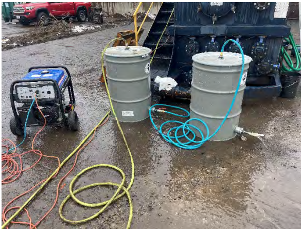
Photo #15 Water treatment system consisting of two 55-gallon activated carbon vessels connected in series.
