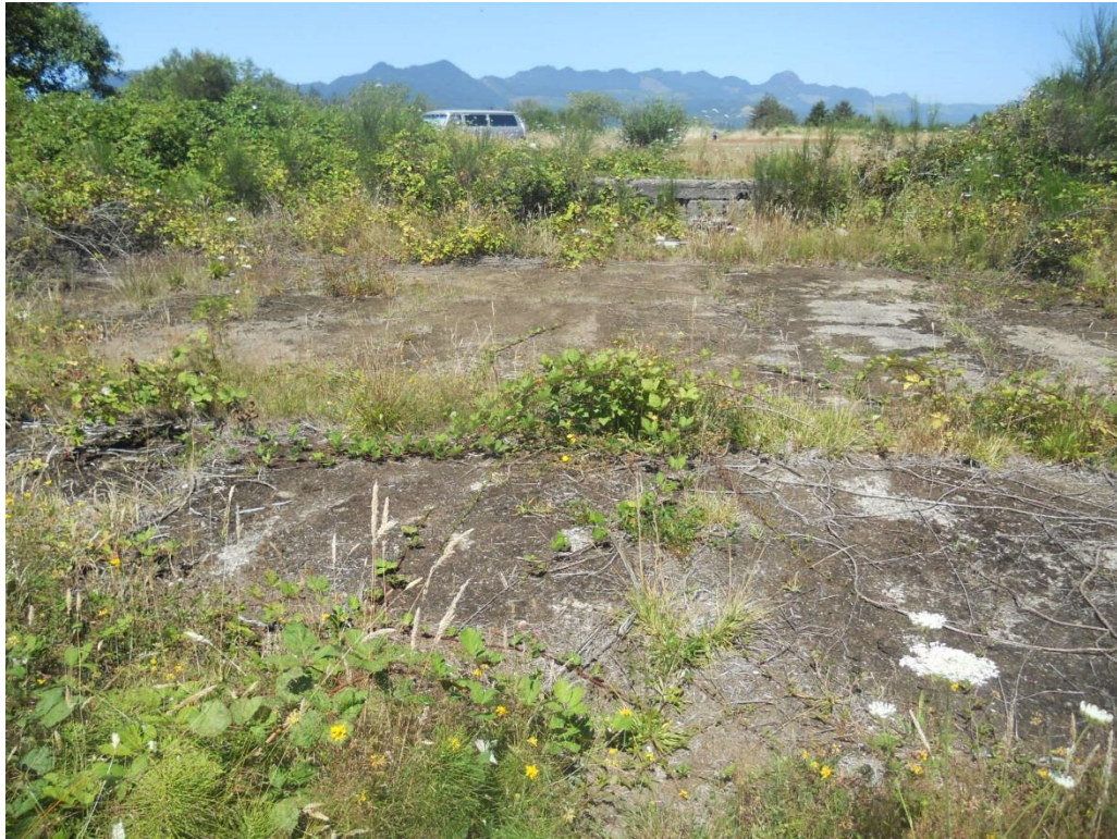
Photo 3. Concrete slab on the southern half of the subject property, facing north.
