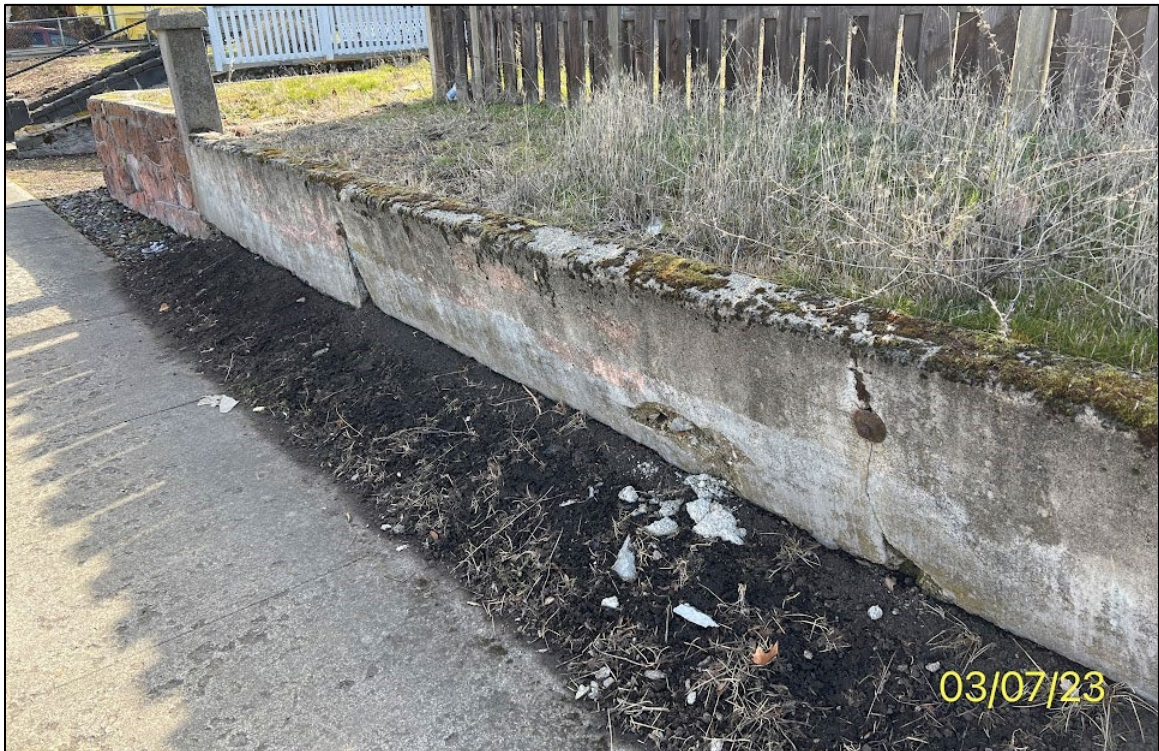
Photo 3: Current conditions of the leaning and cracked retaining wall mentioned above located along East 12 th Street.
