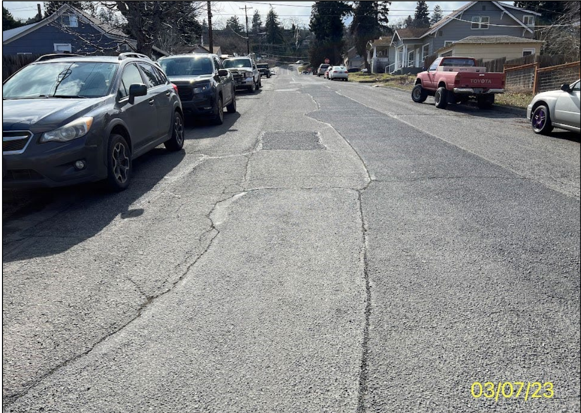
Photo 4: Cracking in the pavement observed along Jefferson Street.
